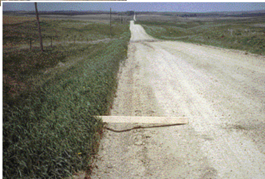
Secondary ditch over six inches deep.
