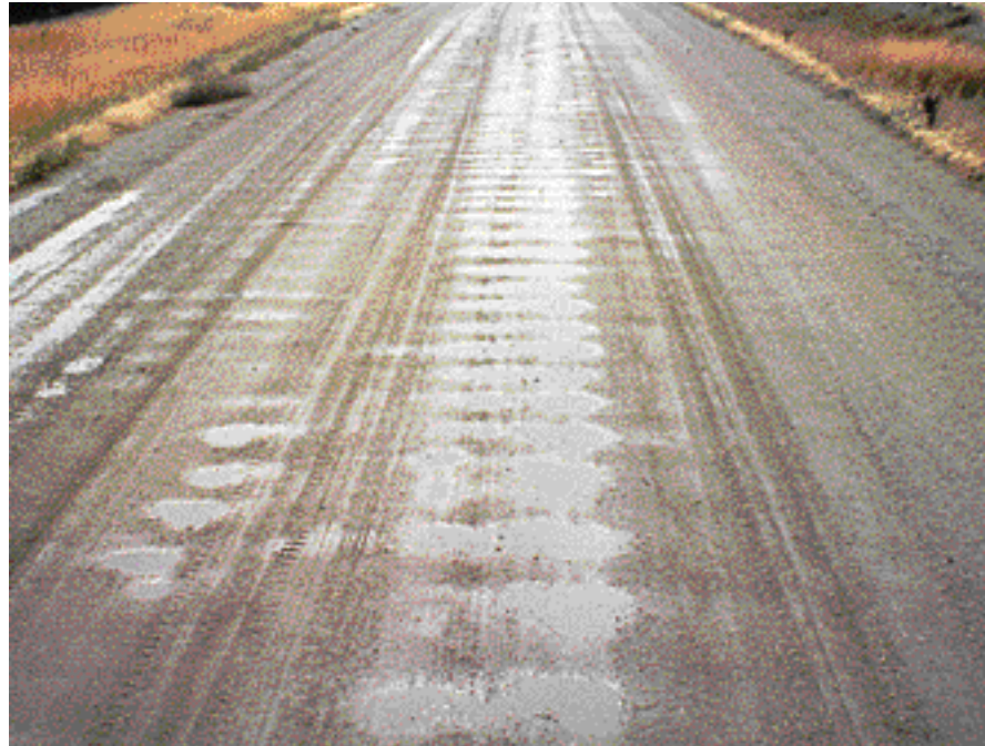
A road that lacks good crown. There is also centerline corrugation (washboarding), a problem that will grow worse when there is inadequate crown.
