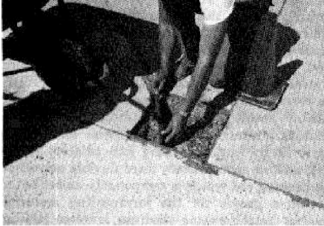
Figure 3. Placement of joint filler sheet to maintain active crack through area to be patched.
