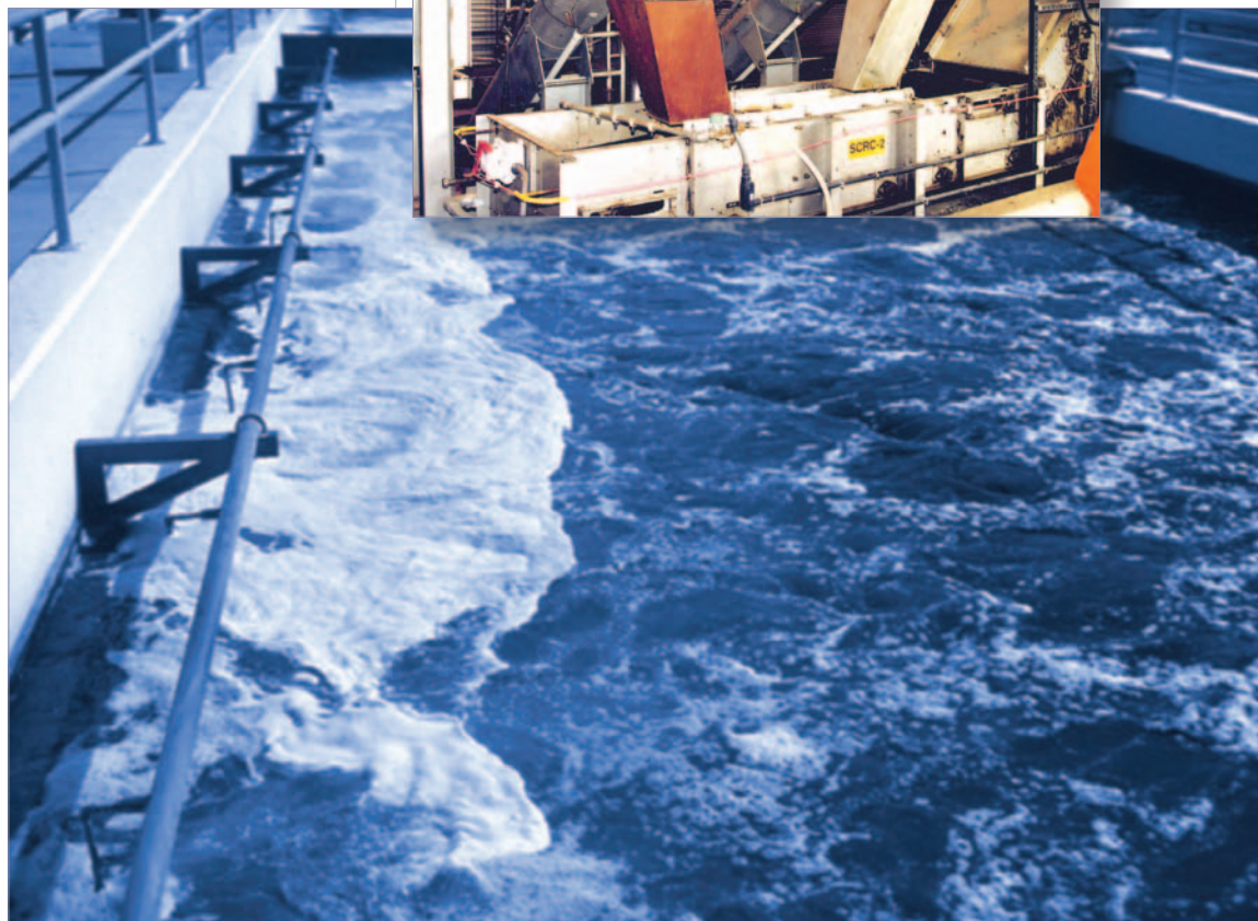
Aerated Grit Chamber
