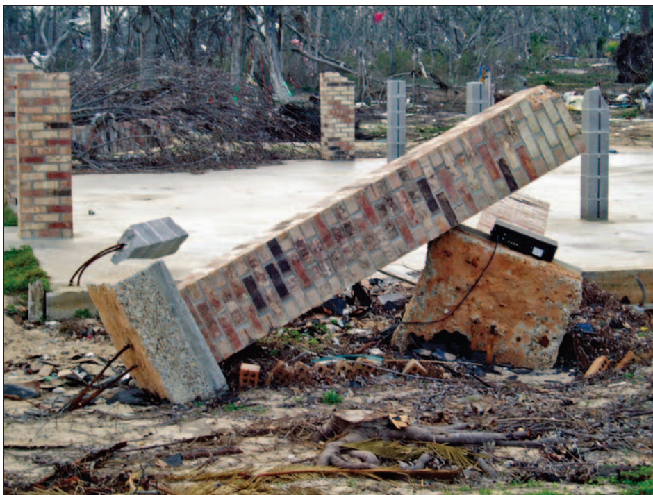
Figure 10-17. Performance comparison of pier foundations: piers on discrete footings (foreground) failed by rotating and overturning while piers on more substantial footings (in this case a concrete mat) survived Hurricane Katrina (Pass Christian, MS, 2005)
