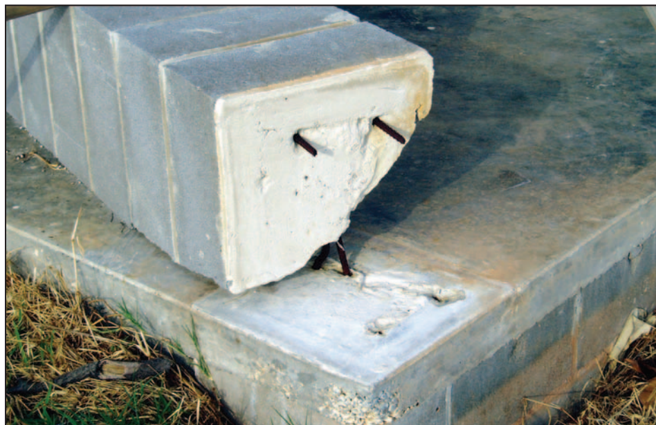
Figure 10-7. Column connection failure, Hurricane Katrina (Belle Fontaine Point, Jackson County, MS, 2005)
