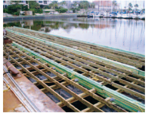
Treated glulams supporting floating dock
