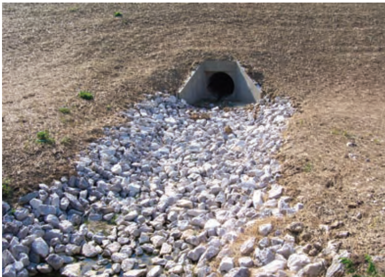
Figure 17. Make sure inlets, outlets, and slopes are well stabilized before leaving the site and filing your "Notice of Termination" for ending permit coverage.
