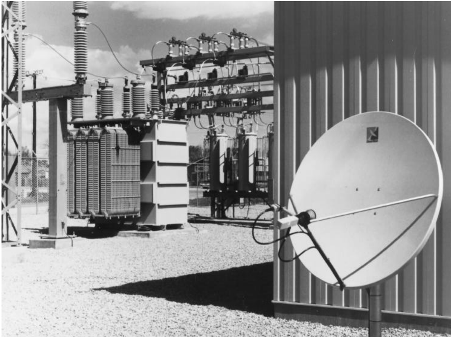
Figure 17-9: VSAT Installed in Electric Substation. Courtesy of Nova Net, Inc.
