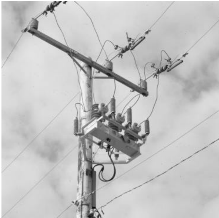
Figure 5-52: Mounted Recloser. Courtesy of Cooper Power Systems.
