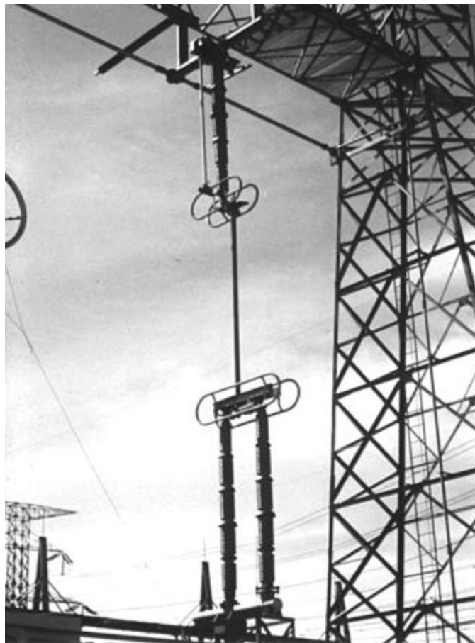
Figure 5-30: Vertical Reach Switch. Courtesy of Southern States, Inc.
