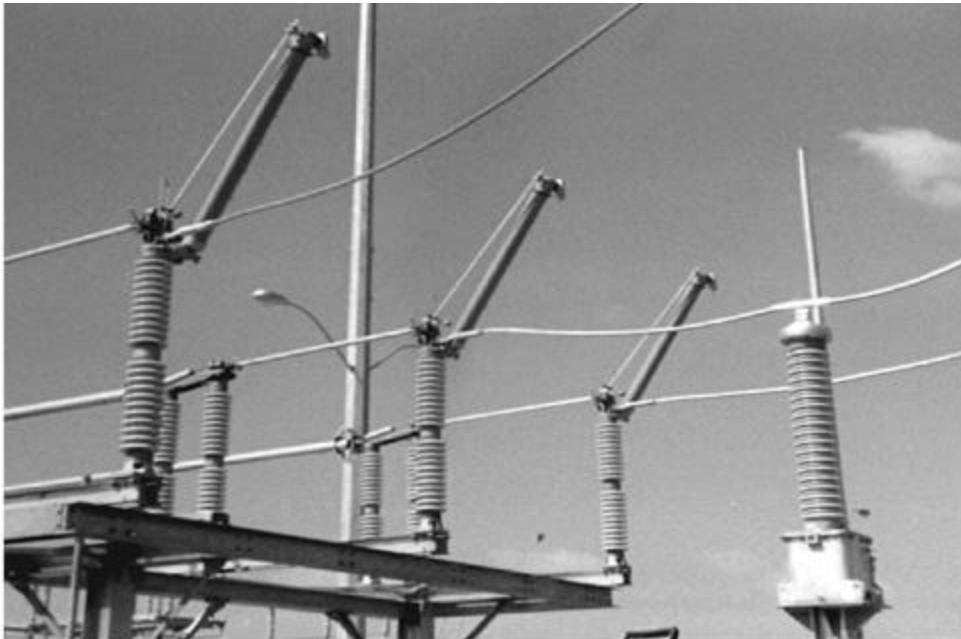
Figure 5-24: Horizontally Mounted Vertical-Break Interrupter Switch. Courtesy of Tuley & Associates, Inc.
