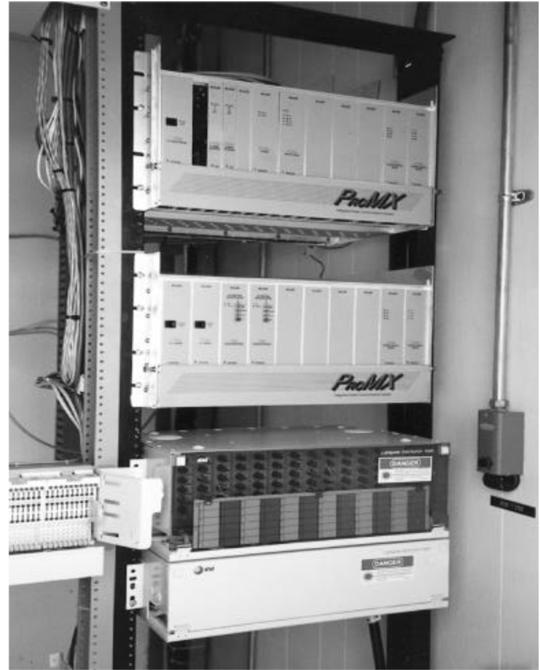
Figure 17-8: Fiber-Optic Multiplexers (Above) and Fiber-Optic Patch Panel (Below)
