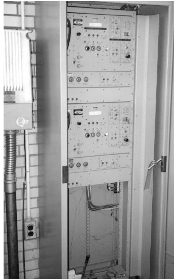
Figure 16-5: 19-Inch Rack-Mount Relay/ Communications Equipment (PSI)
