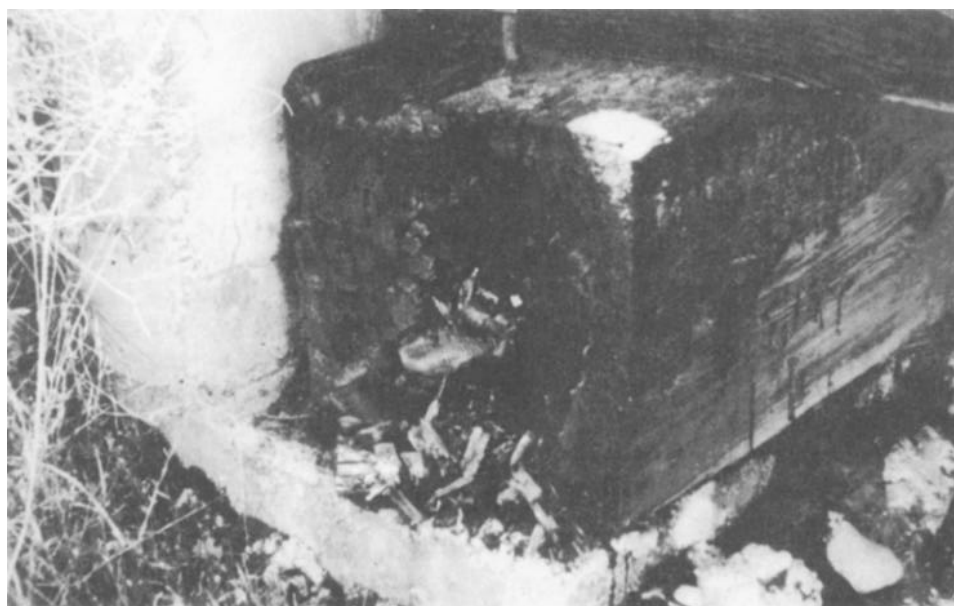
Figure 5-14. Advanced wood decay in crosstie.
