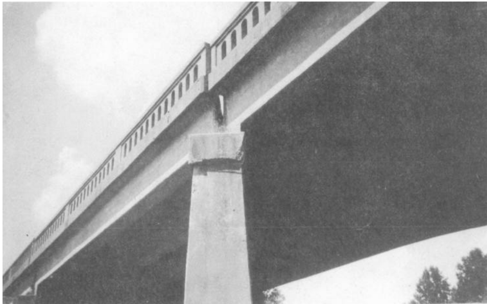
Figure 5-21. Differential pier movement causing superstructure movement.
