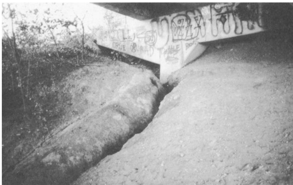
Figure 5-25. Embankment erosion due to improper drainage. (Sheet 2 of 2)
