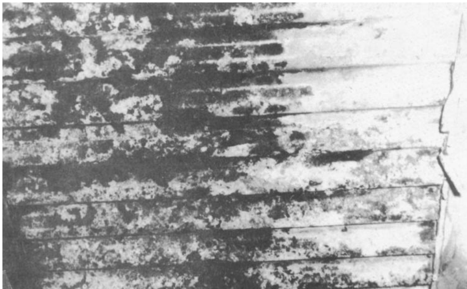
Figure 8-29. Rusted stay-in-place forms underneath a concrete deck.
