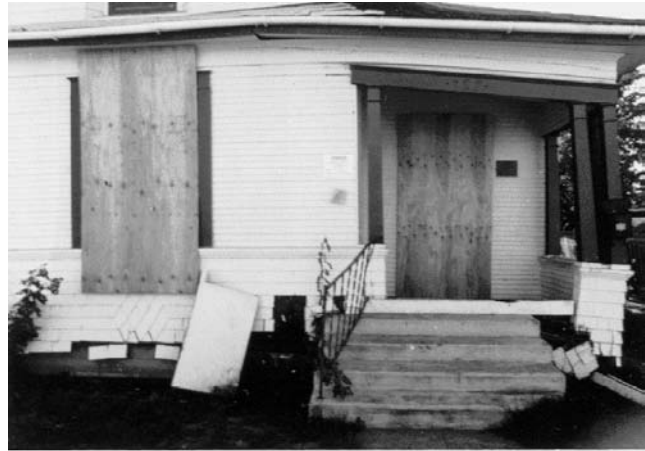
Figure 10 - This home wasn't bolted and slid off its foundation. Sometimes the damage can be so bad that houses have to be demolished.
