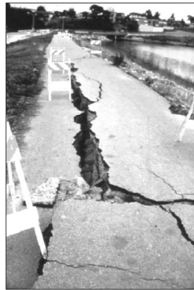
Figure 35 - Lateral Spreading, Loma Prieta Earthquake, October 17, 1989. Lateral spreading damaged levee road along the San Lorenzo River.
