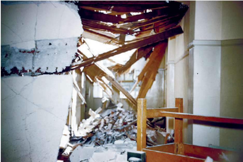
Figure 4-17: Destroyed exit corridor, Bakersfield, Kern County, CA, 1952
