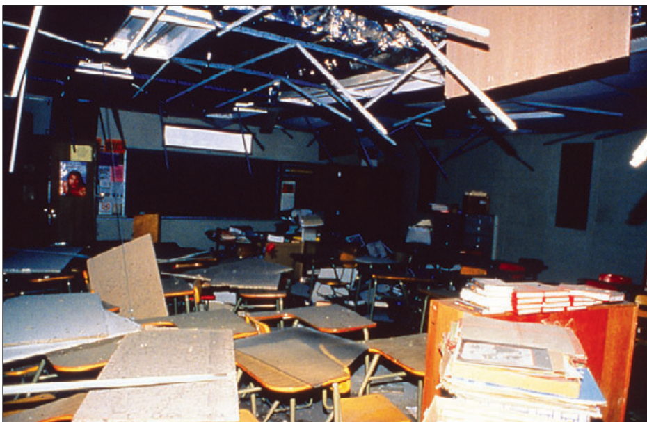
Figure 4-25: Ceiling damage, Northridge, CA, 1994
