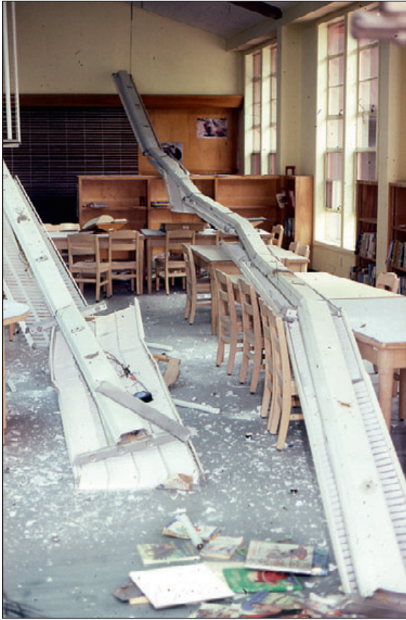
Figure 4-10: Fallen light fixtures, library, Coalinga, CA, 1983
