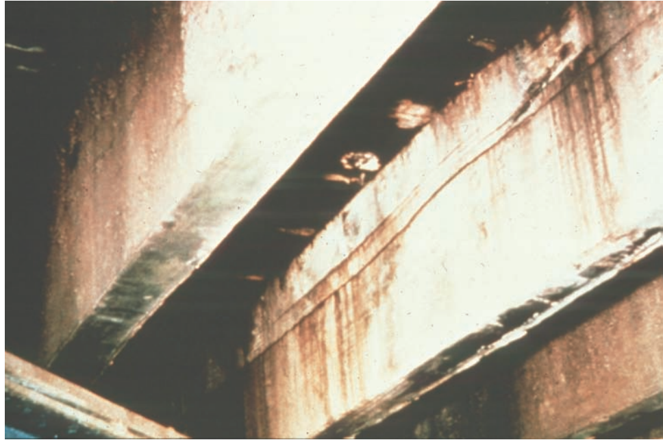
Figure 6.1.12 Horizontal Shear Crack in a Timber Beam
