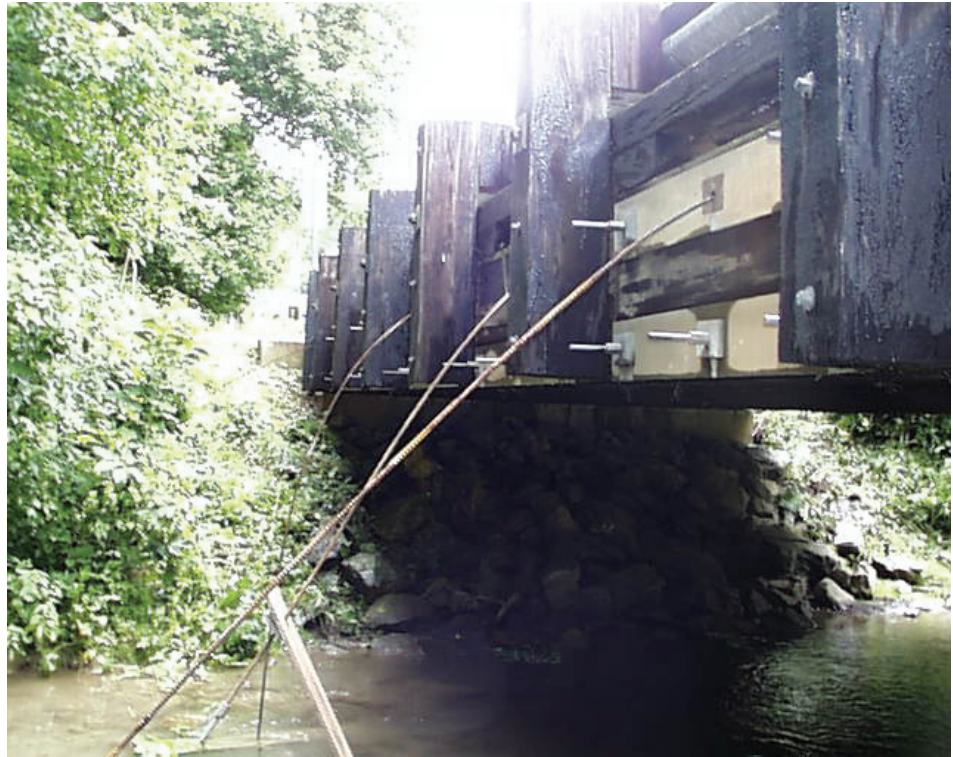
Figure 6.3.10 Broken Stressing Rods
