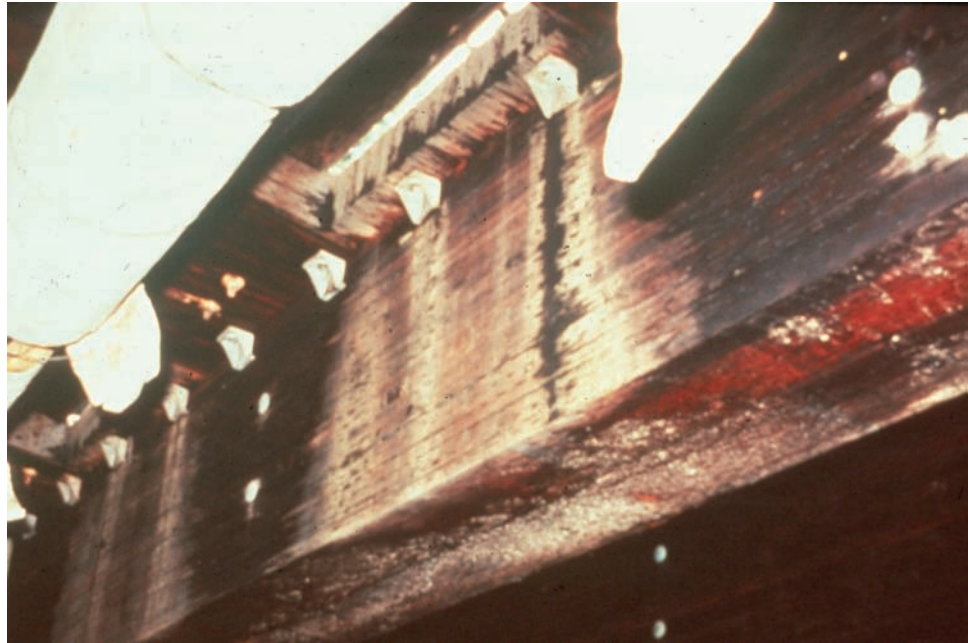
Figure 6.2.12 Decay on Glulam Beam
