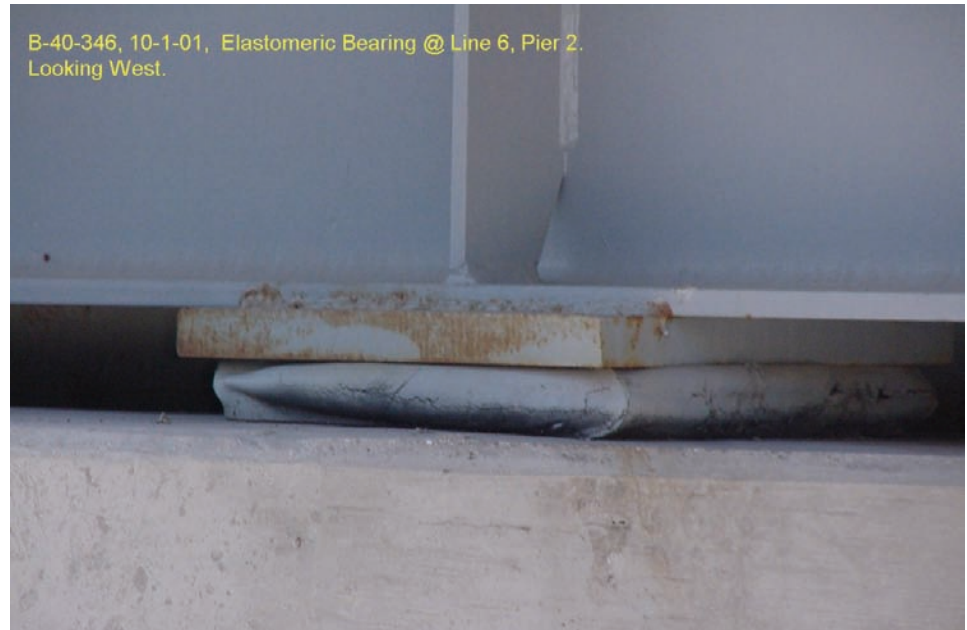
Figure 9.1.35 Neoprene Bearing Pad Excessive Bulging
