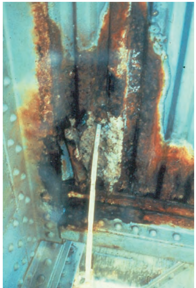
Figure 5.2.12 Deteriorated Stay-in-Place Form
