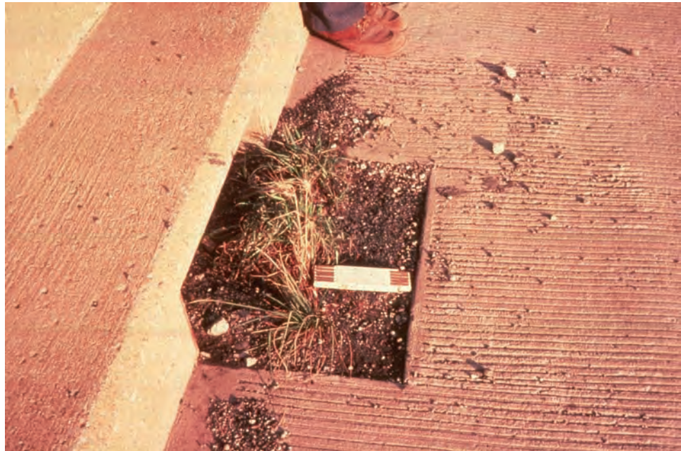
Figure 5.4.21 Clogged Drainage Inlet
