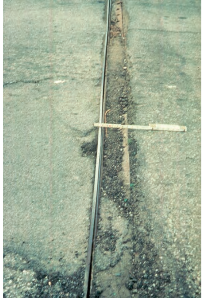
Figure 5.4.15 Debris Lodged in a Sliding Plate Joint
