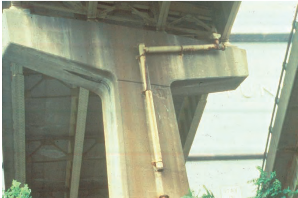
Figure 5.4.14 Downspout Pipes and Cleanout Plugs
