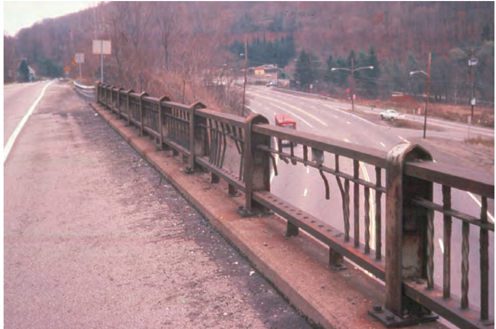
Figure 5.5.10 Damaged Steel Post Bridge Railing
