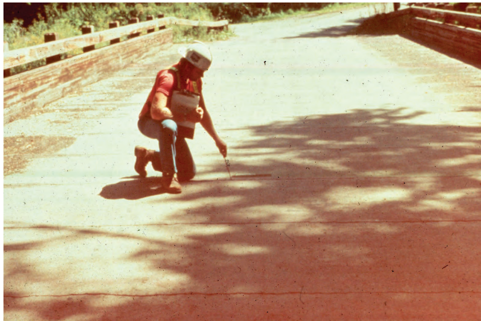
Figure 5.1.7 Inspector Probing Timber with a Pick at Reflective Cracks in the Asphalt Wearing Surface
