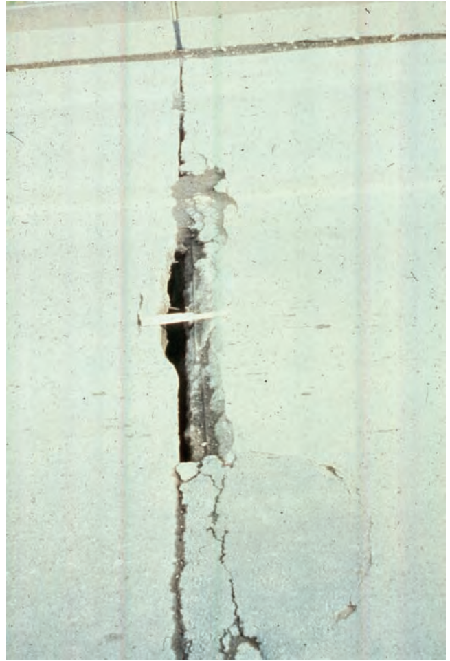
Figure 5.4.18 Failed Compression Seal
