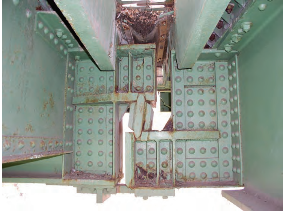
Figure 5.4.22 Drainage Trough with Debris Accumulation
