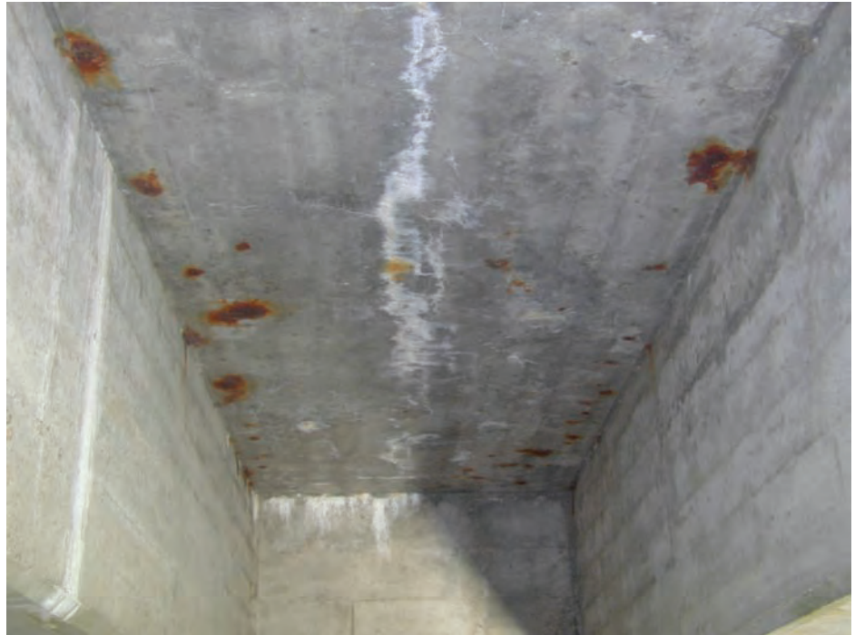
Figure 5.2.11 Underside View of Longitudinal Deck Crack
