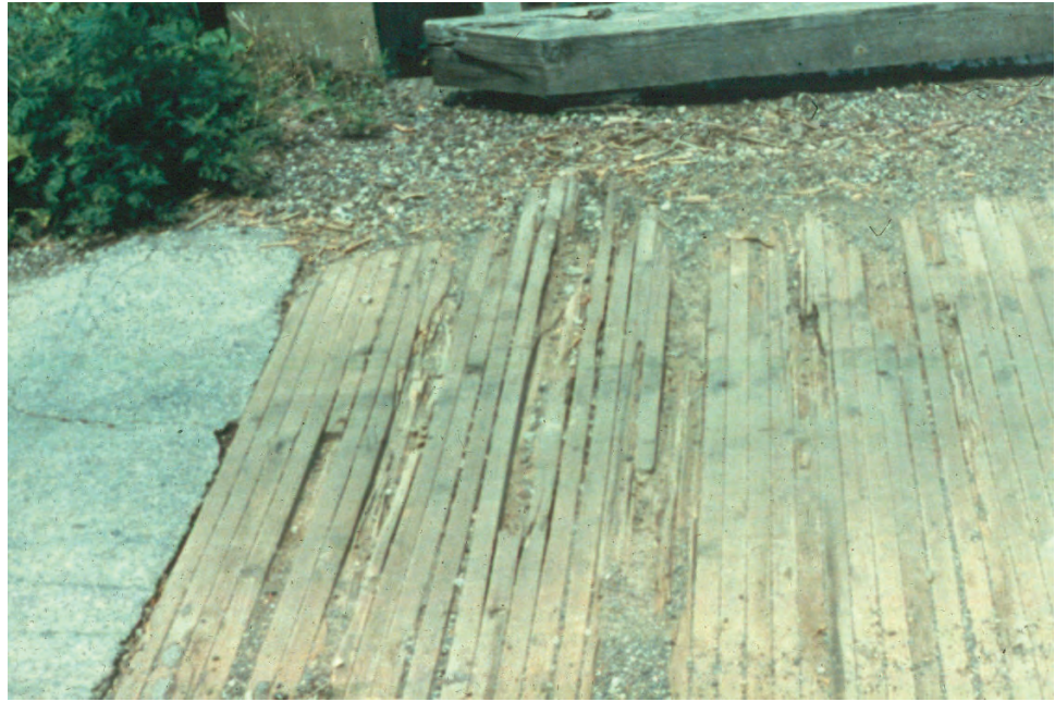
Figure 5.1.8 Wear and Weathering on a Timber Deck
