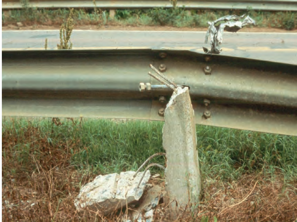
Figure 5.5.11 Approach Guardrail Collision Damage
