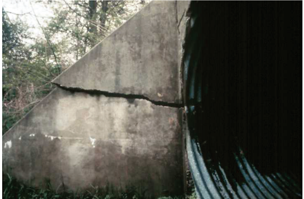
Figure P.3.23 Cracking of Culvert End Treatment Due to Foundation Settlement
