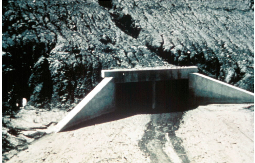
Figure P.3.28 Slide Failure
