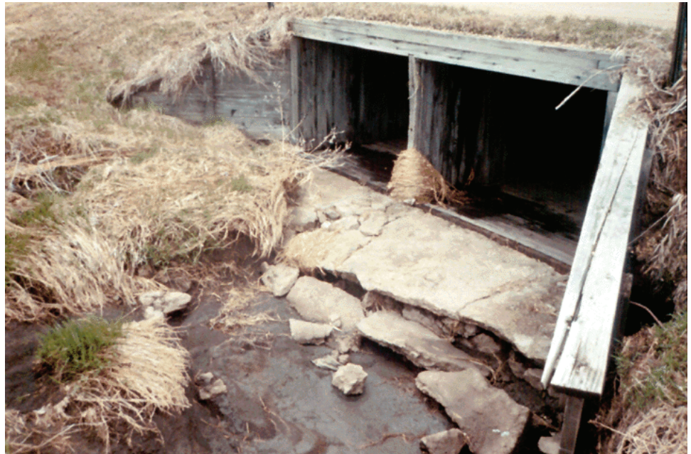
Figure P.3.24 Scour and Undermining at Culvert Inlet
