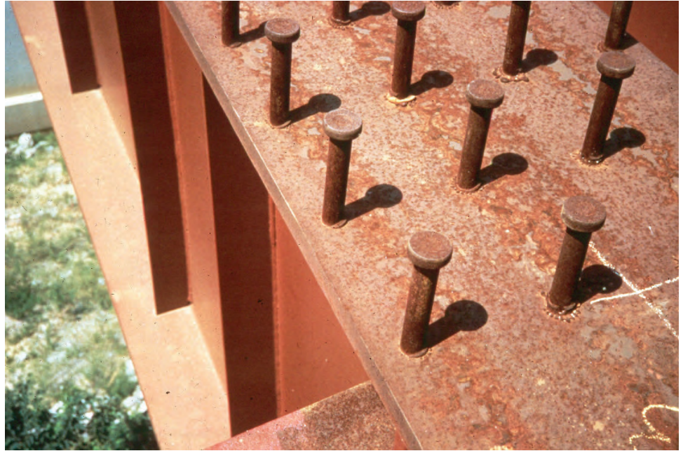
Figure P.1.27 Shear Studs on Top Flange of Girder (before Concrete Deck is Placed)
