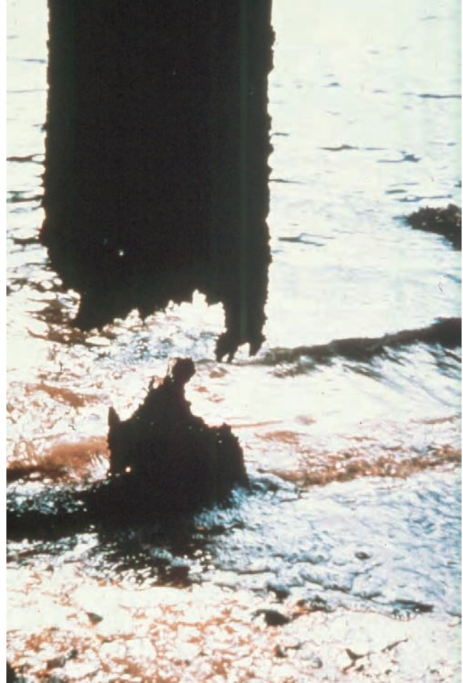
Figure 10.2.50 Timber Bent Damage due to Shipworm Marine Borers
