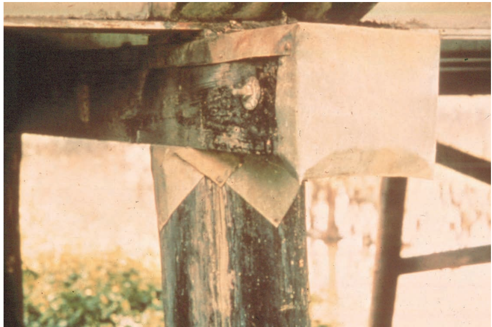
Figure 10.2.45 Decay in Timber Bent Cap (Note “Protective” Cover / Flashing)
