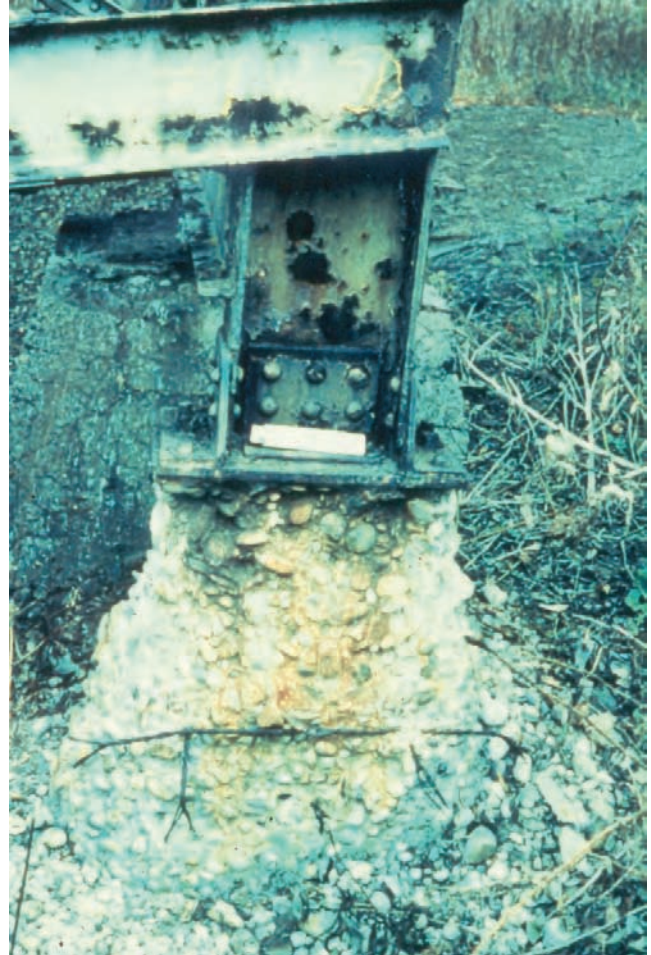
Figure 10.2.40 Deterioration of Concrete Pedestal Supporting Steel Column
