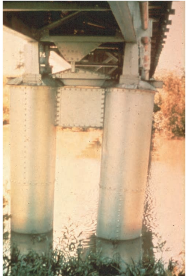
Figure 10.2.35 Tipping of Bent due to Scour/Undermining
