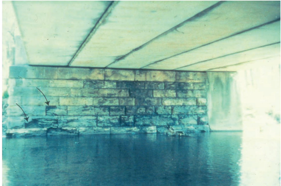
Figure 10.2.51 Deteriorated and Missing Stone at Masonry Pier
