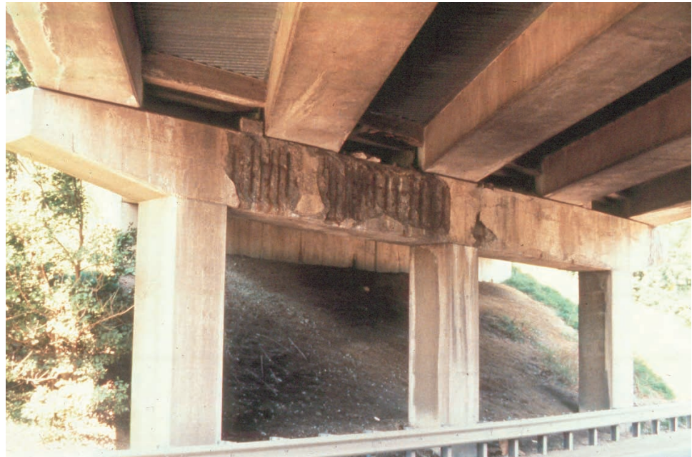
Figure 10.2.38 Severe Concrete Spalling on Bent Cap
