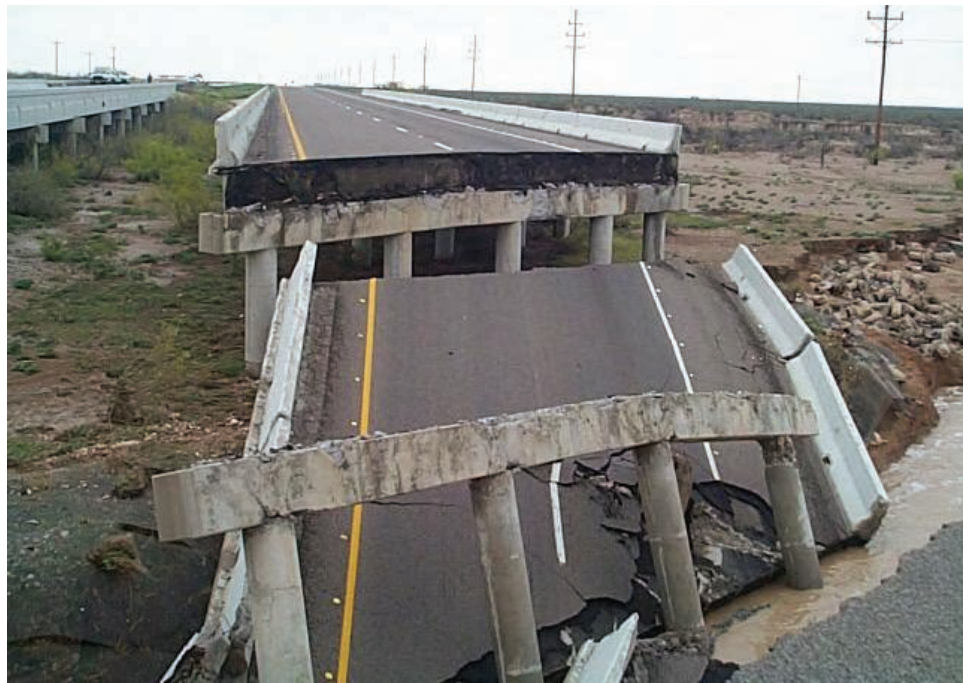
Figure 10.2.34 Pier Movement and Superstructure Damage due to Scour/Undermining
