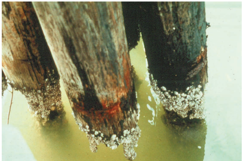
Figure 10.2.49 Timber Pile Damage due to Limnoria Marine Borers
