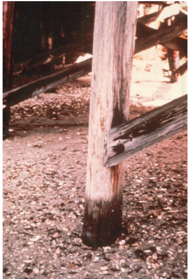
Figure 10.2.47 Decay of Timber Bent Column at Ground Line
