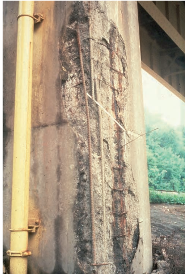
Figure 10.2.36 Concrete Deterioration due to Contaminated Drainage
