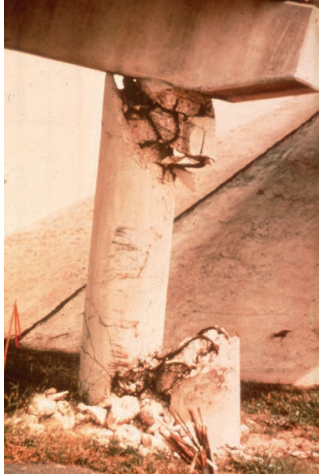
Figure 10.2.39 Collision Damage to Pier Column
