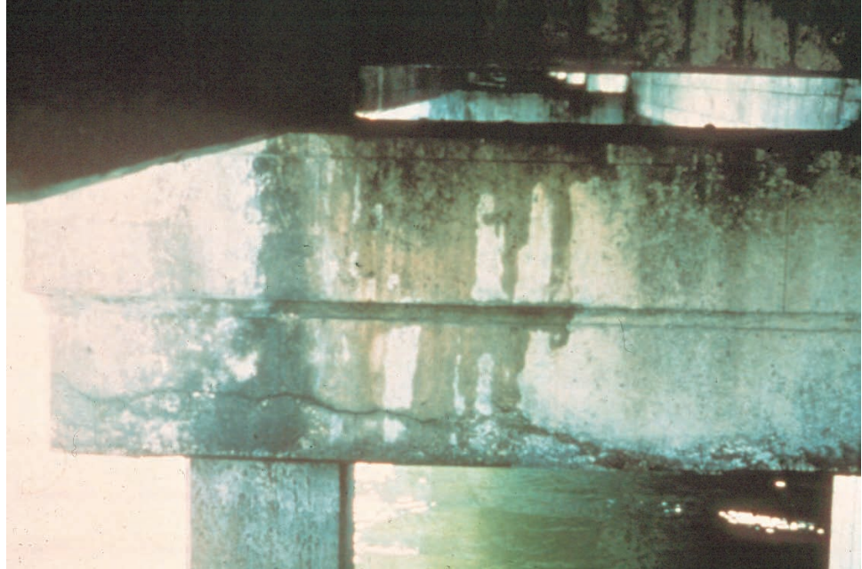
Figure 10.2.37 Crack in Concrete Bent Cap
