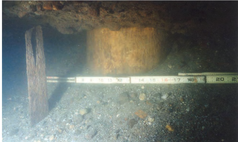
Figure 11.3.25 Pier Undermining, Exposing Timber Foundation Pile
