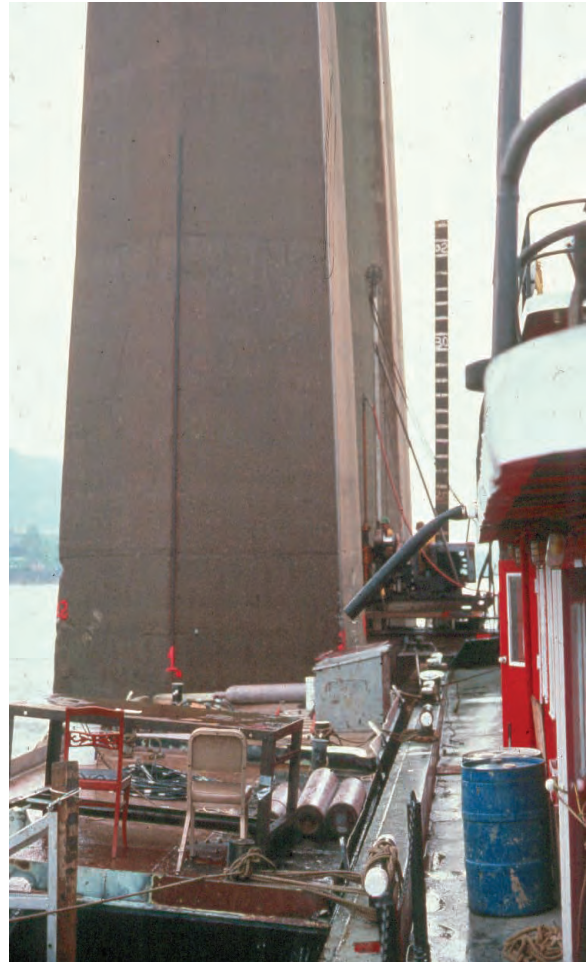
Figure 11.3.10 Permanent Reference Point (Bolt Anchored in Nose of the Pier, Painted Orange)
