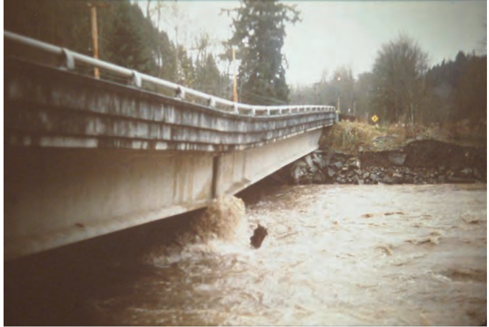
Figure 11.3.14 Movement of a Substructure Unit
