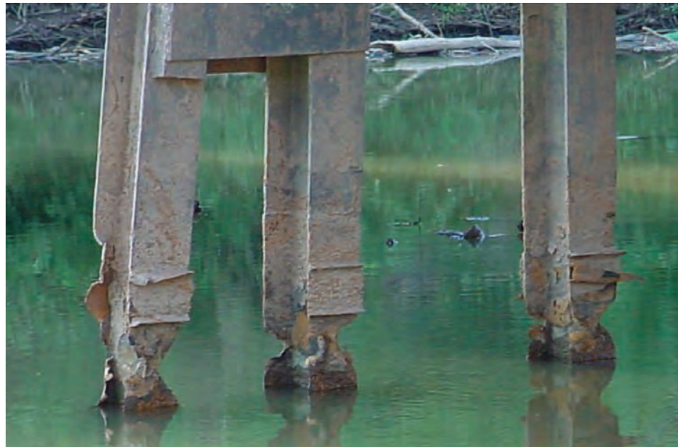
Figure 11.3.28 Deteriorated Steel Piles at Splash Zone
