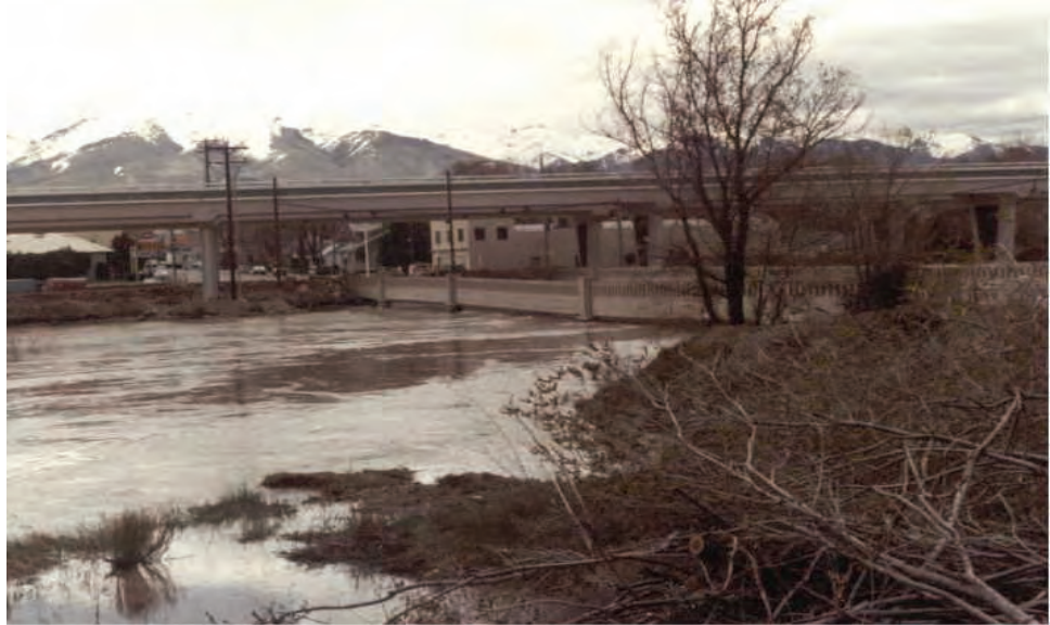
Figure 11.3.12 Flood Conditions: Note Pier Settlement.
