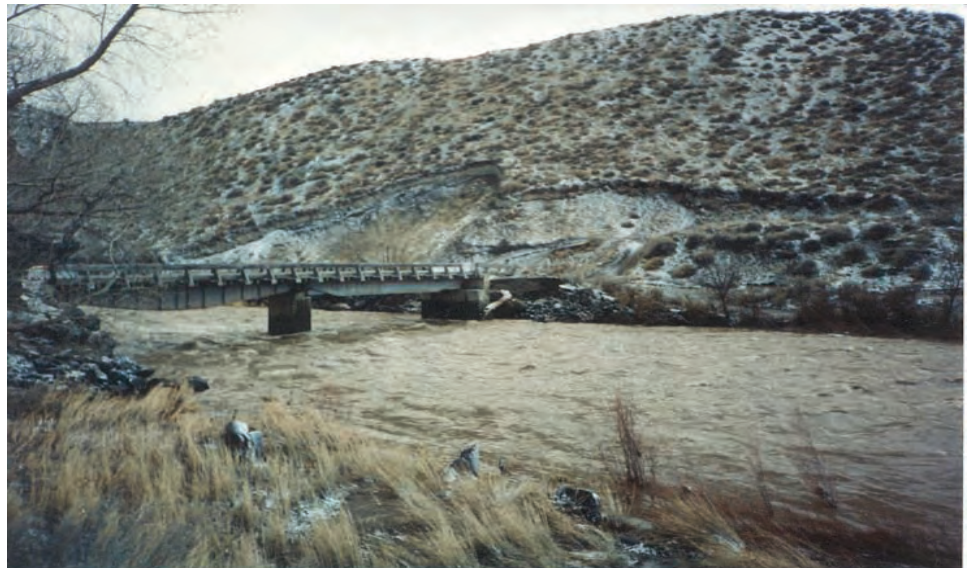
Figure 11.3.21 Severe Flood-Induced Abutment Scour
