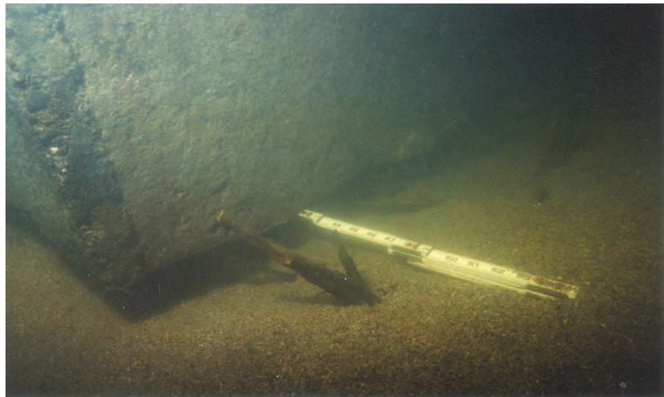
Figure 11.3.11 Local Scour; Causing Undermining of a Pier
