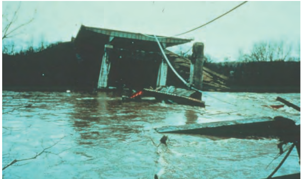
Figure 11.3.1 Schoharie Creek Bridge Failure
