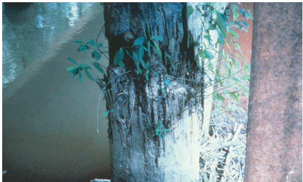
Figure 11.3.27 Deteriorated Timber Piling
