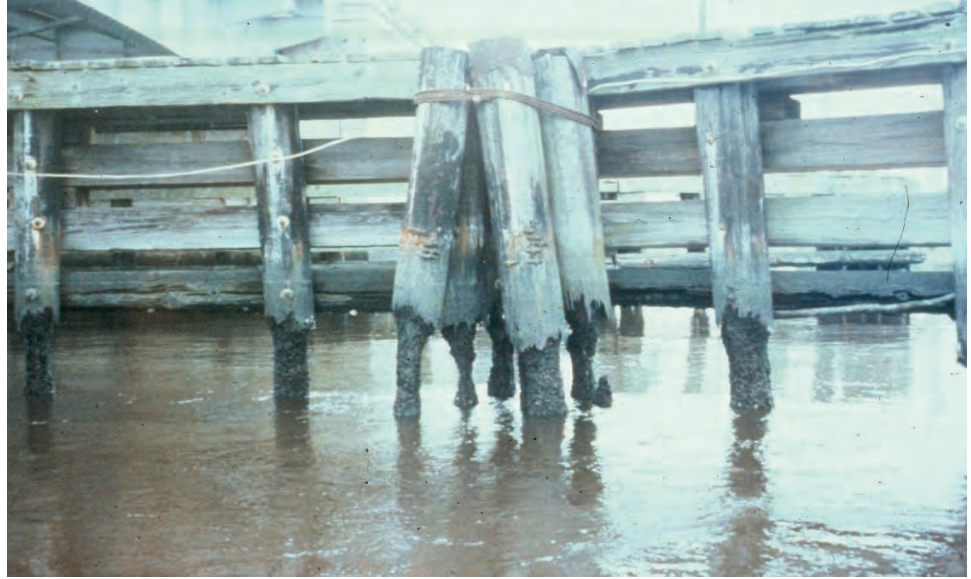
Figure 11.3.23 Damaged Protective System
