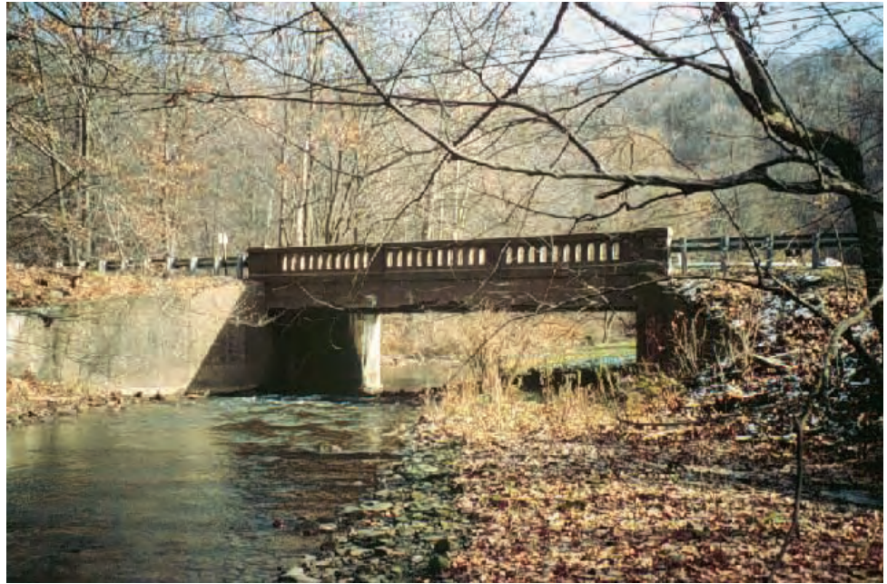
Figure 11.2.50 Stream Alignment Not Parallel with Abutments
