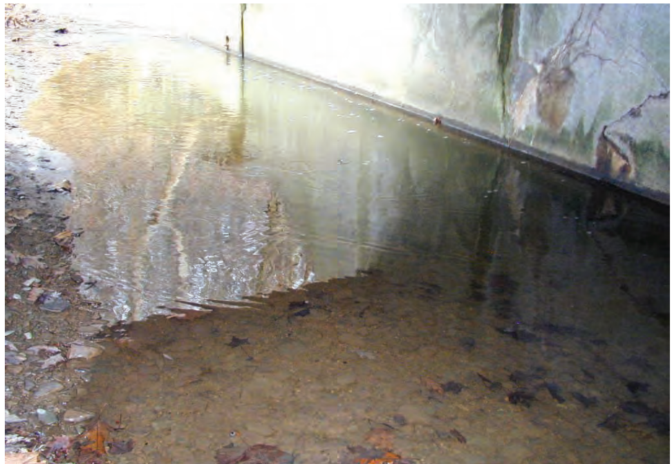
Figure 11.2.13 Local Scour at an Abutment
