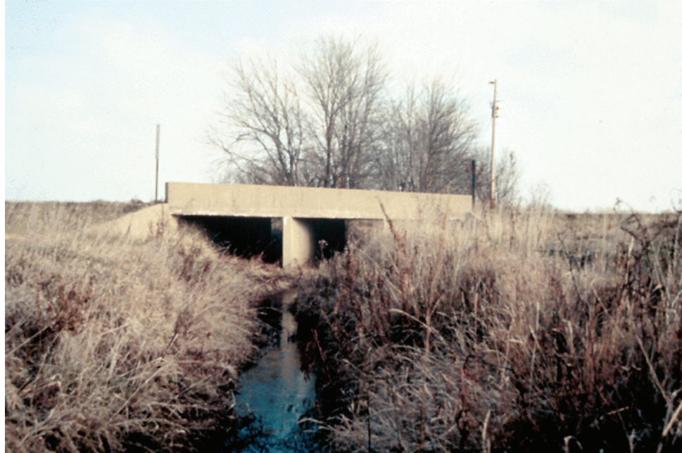
Figure 11.2.8 Vegetation Constricting the Waterway
