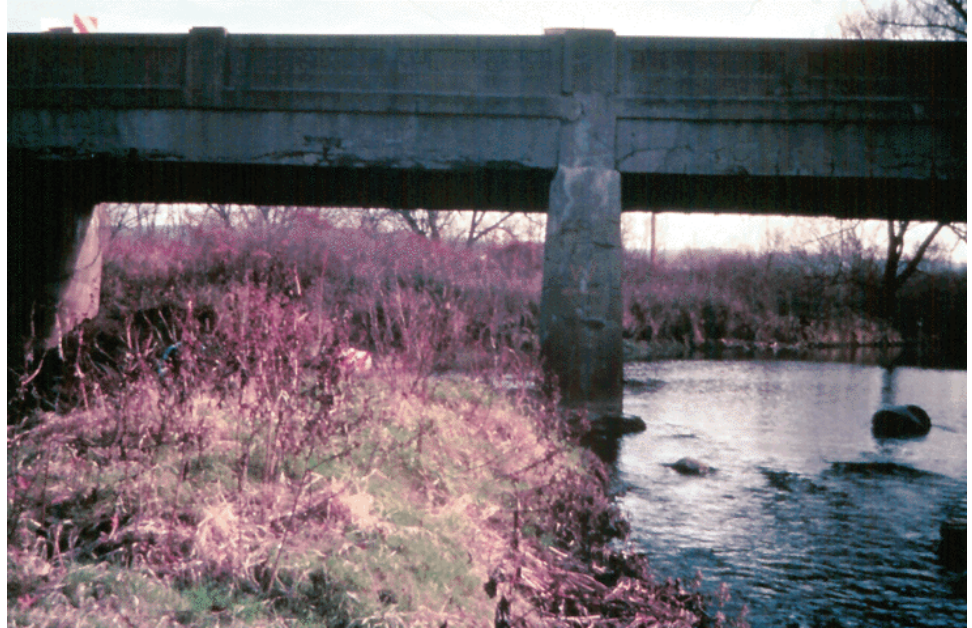
Figure 11.2.47 Typical Misaligned Waterway
