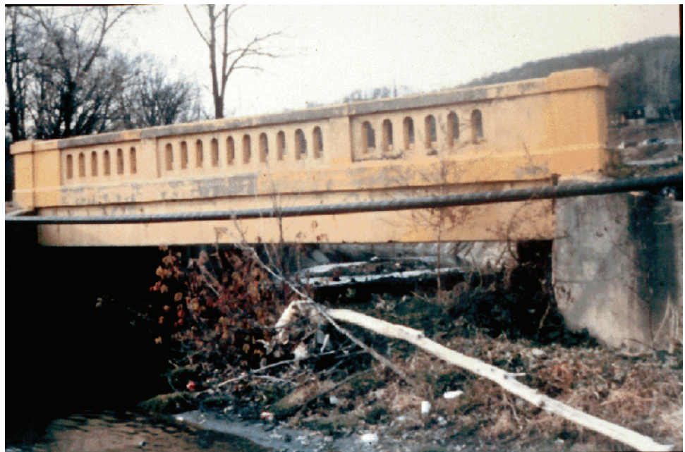
Figure 11.2.42 Debris and Sediment in the Downstream Channel
