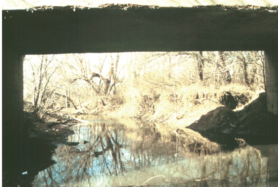
Figure 11.2.37 Unstable, Sloughing Banks
