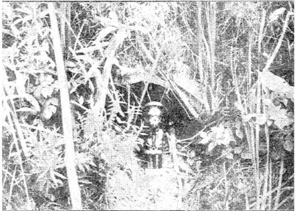
Figure 11.2.58 (Exhibit 64) Culvert Almost Completely Blocked by Sediment Accumulation
