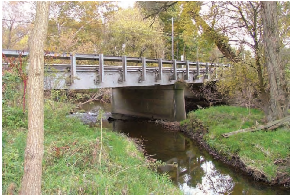
Figure 11.2.38 Sediment Accumulation Redirecting Streamflow
