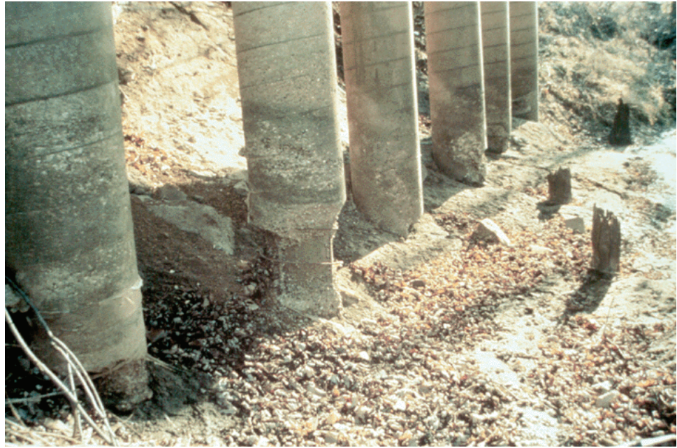
Figure 11.2.28 Pile Bent Deterioration Normally Hidden Underwater
