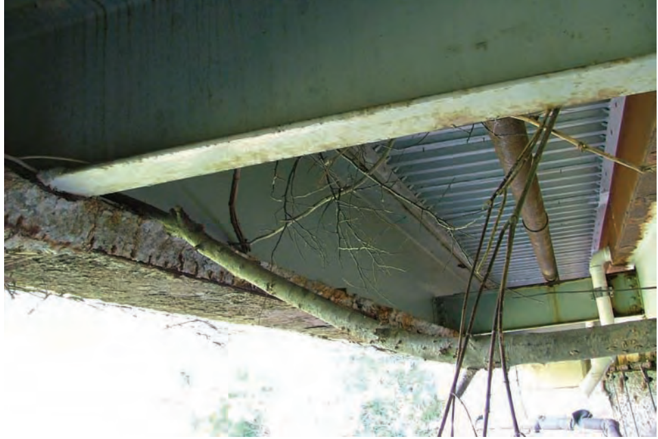
Figure 11.2.31 Drift Lodged in a Superstructure
