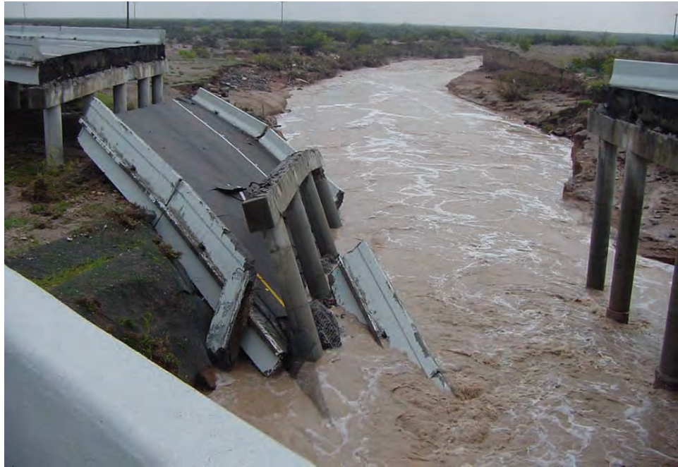
Figure 11.1.1 Pier Foundation Failure
