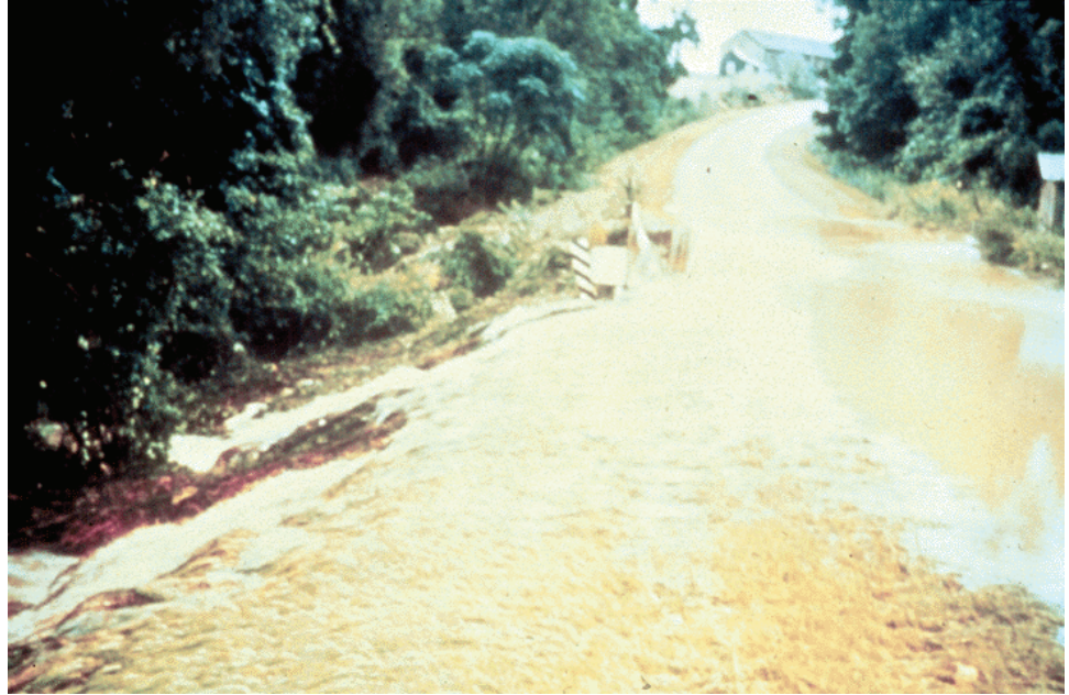
Figure 11.2.57 (Exhibit 63) Culvert Failure Due to Overtopping
