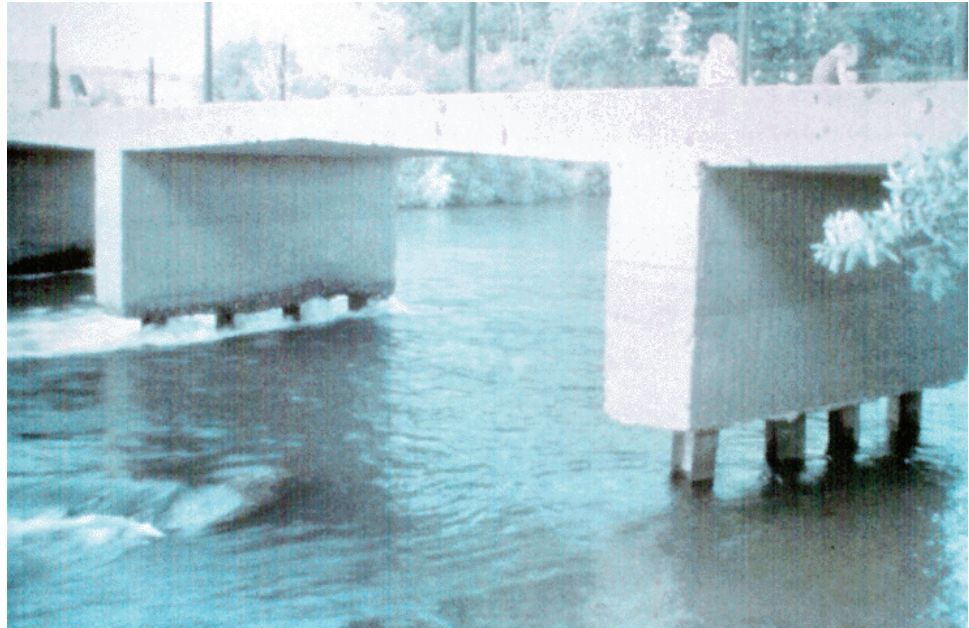
Figure 11.2.52 Exposed Piling Due to Scour
