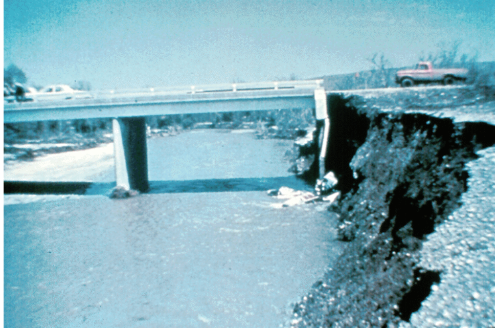
Figure 11.2.17 Lateral Stream Migration Endangering a Full Height Abutment
