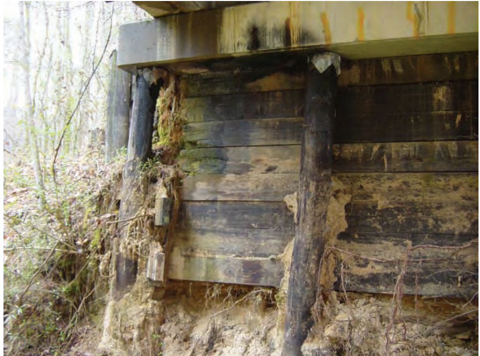
Figure 11.2.44 Scour at a Pile Abutment
