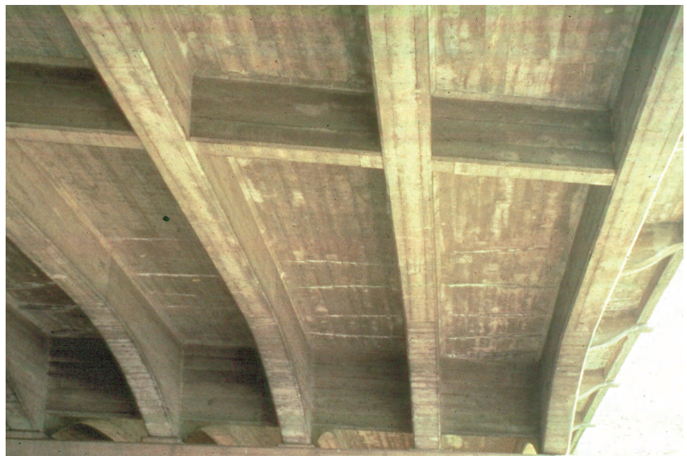
Figure 7.2.14 Flexure Cracks in Tee Beam Deck
