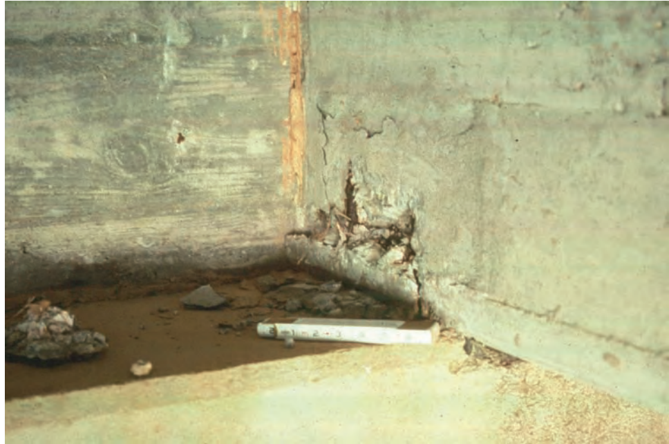
Figure 7.2.10 Deteriorated Tee Beam Bearing Area
