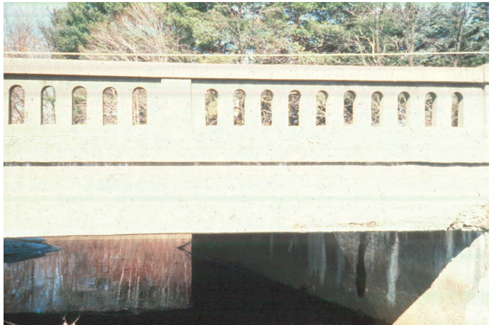
Figure 7.2.19 Deteriorated Tee Beam End Due to Drainage
