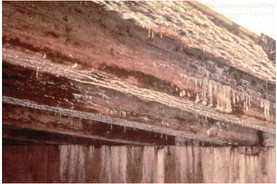
Figure 7.2.15 Stem of a Cast-in-Place Concrete Tee Beam with Contaminated Concrete
