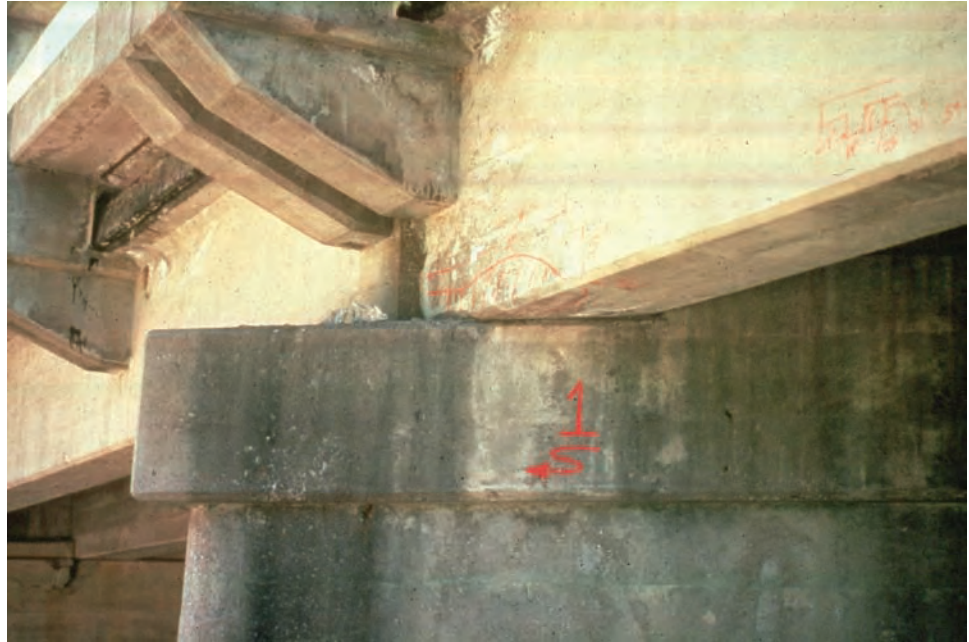
Figure 7.2.12 Shear Zone of Cast-in-Place Concrete Tee Beam Bridge
