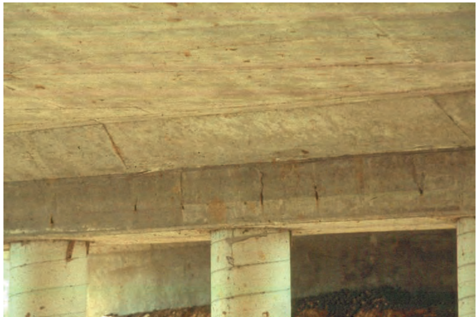
Figure 7.1.6 Shear Zone on the Underside of a Continuous Slab Bridge Near a Pier
