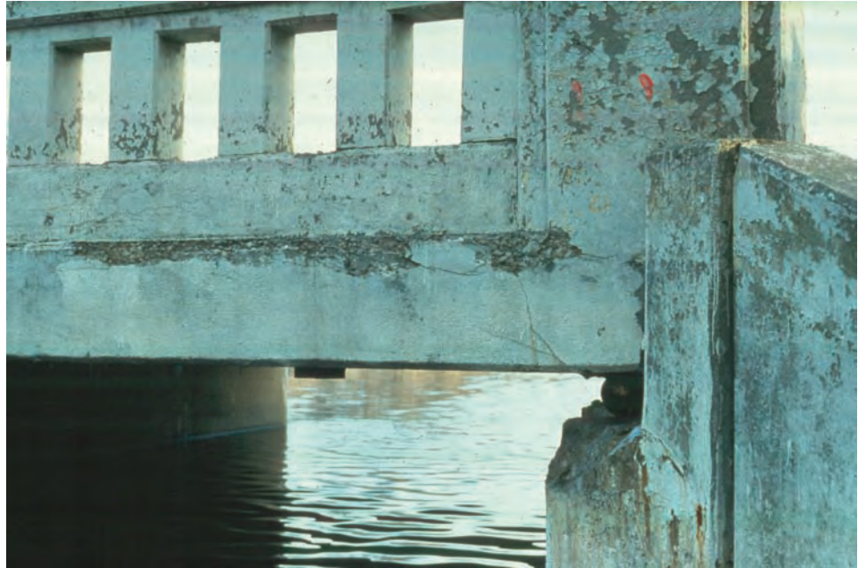
Figure 7.1.5 Shear Cracks in the Ends of a Slab Bridge
