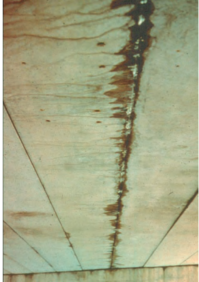
Figure 7.7.4 Leaking Joint between Adjacent Slab Units
