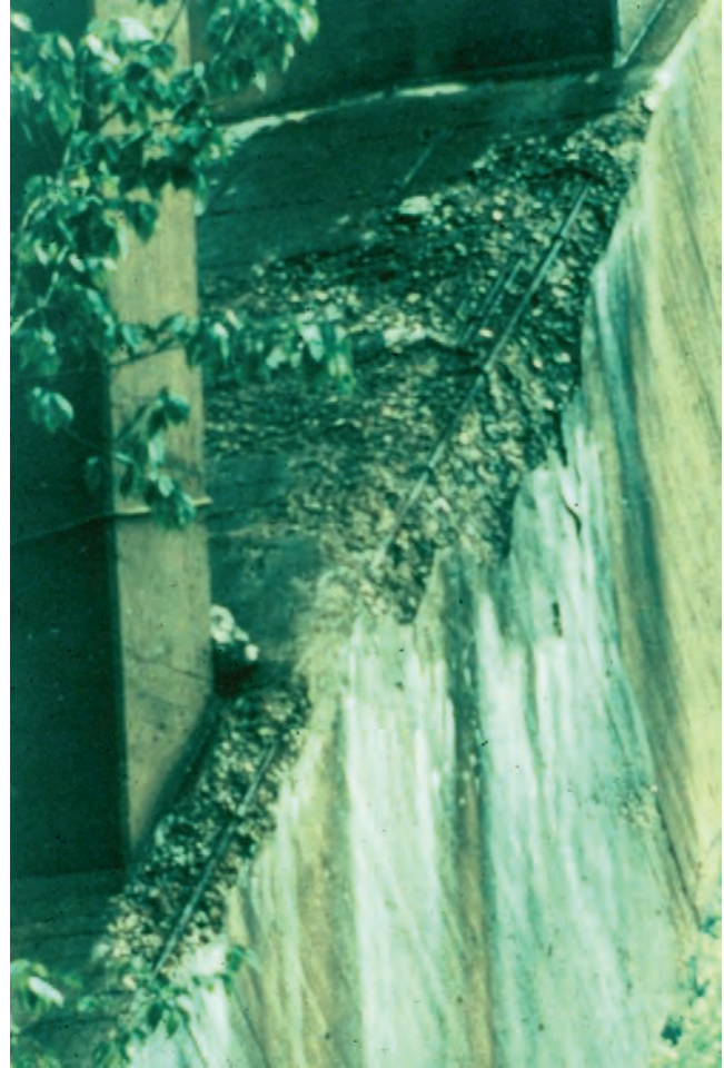
Figure 7.5.18 Scaling and Contamination on an Arch Rib Due to a Failed Drainage System
