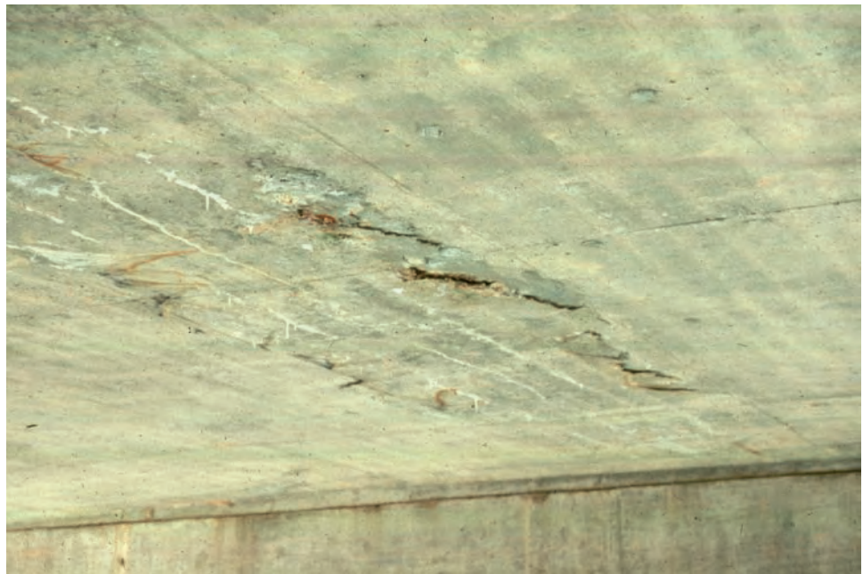
Figure 7.1.7 Concrete Slab Tension Zone: Delamination, Efflorescence, Rust, and Stains
