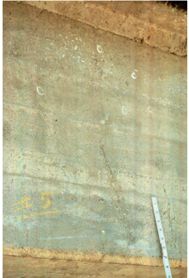
Figure 7.2.13 Flexure Cracks on a Tee Beam
