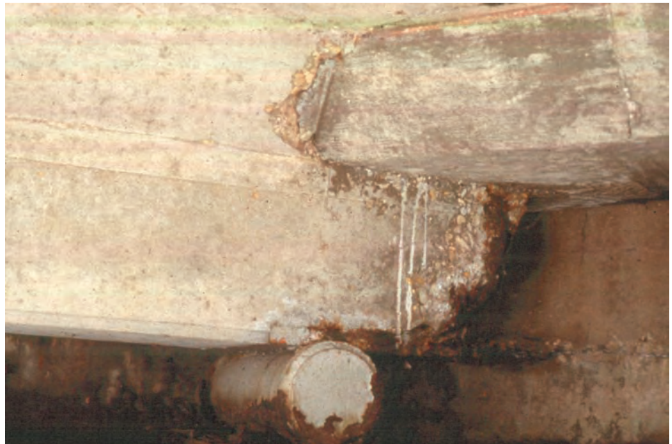
Figure 7.2.9 Spalled Tee Beam End
