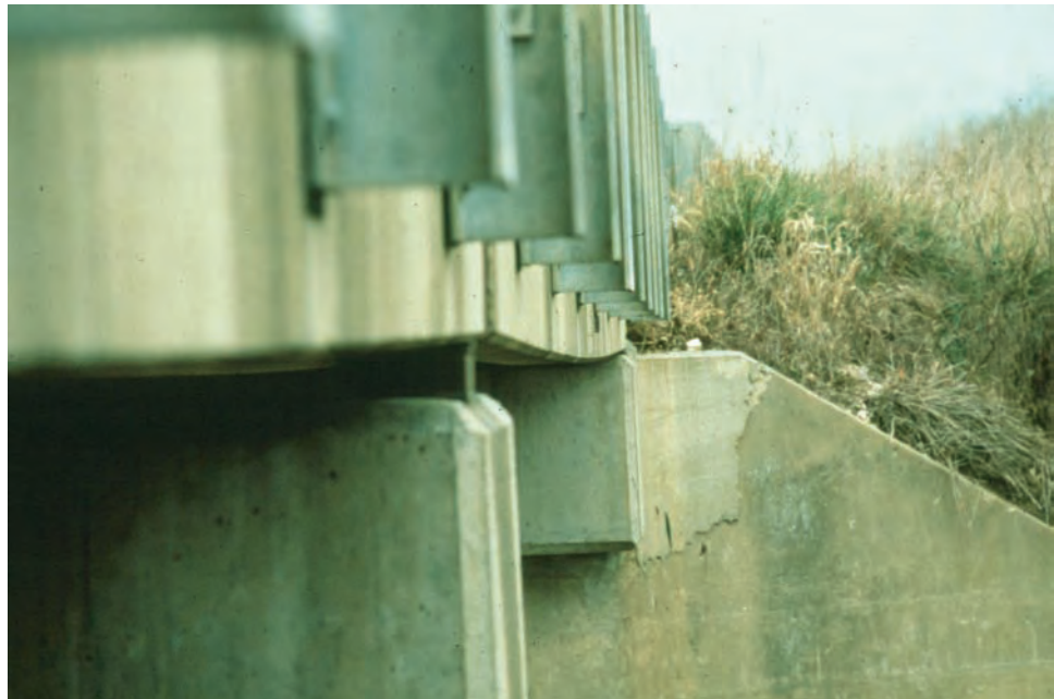
Figure 7.4.5 Excessive Deflection at Midspan
