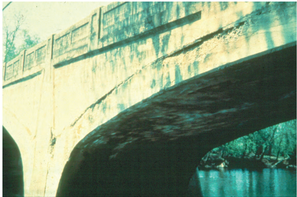
Figure 7.5.16 Deteriorated Arch/Spandrel Wall Interface
