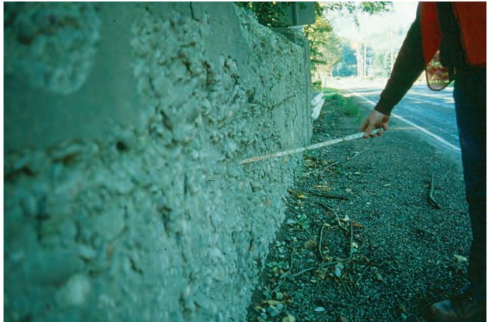
Figure 7.3.9 Close-up of an Interior Face of a Through Girder with Heavy Scaling due to Deicing Agents
