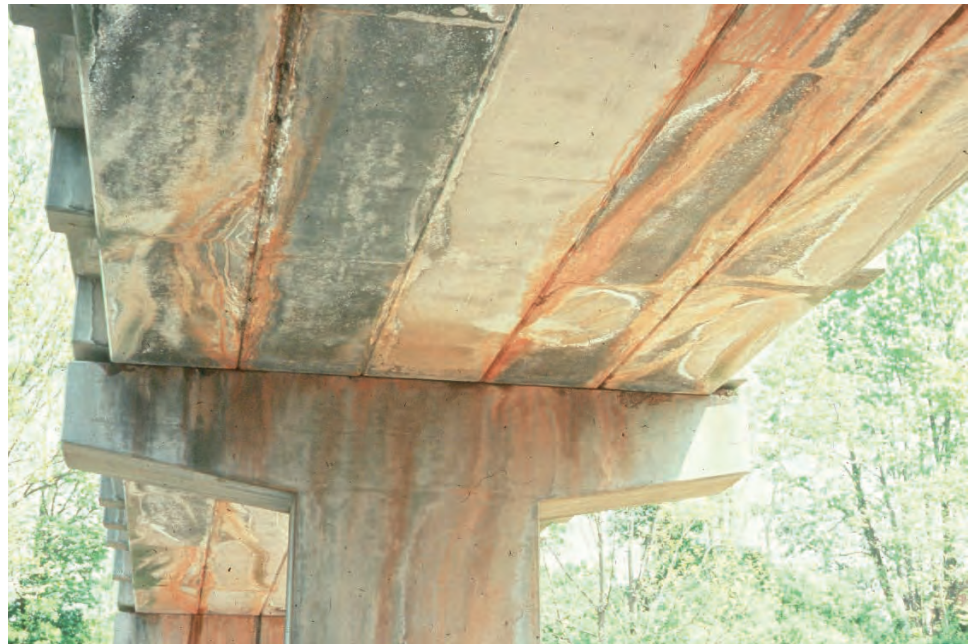
Figure 7.10.16 Joint Leakage and Rust Stain
