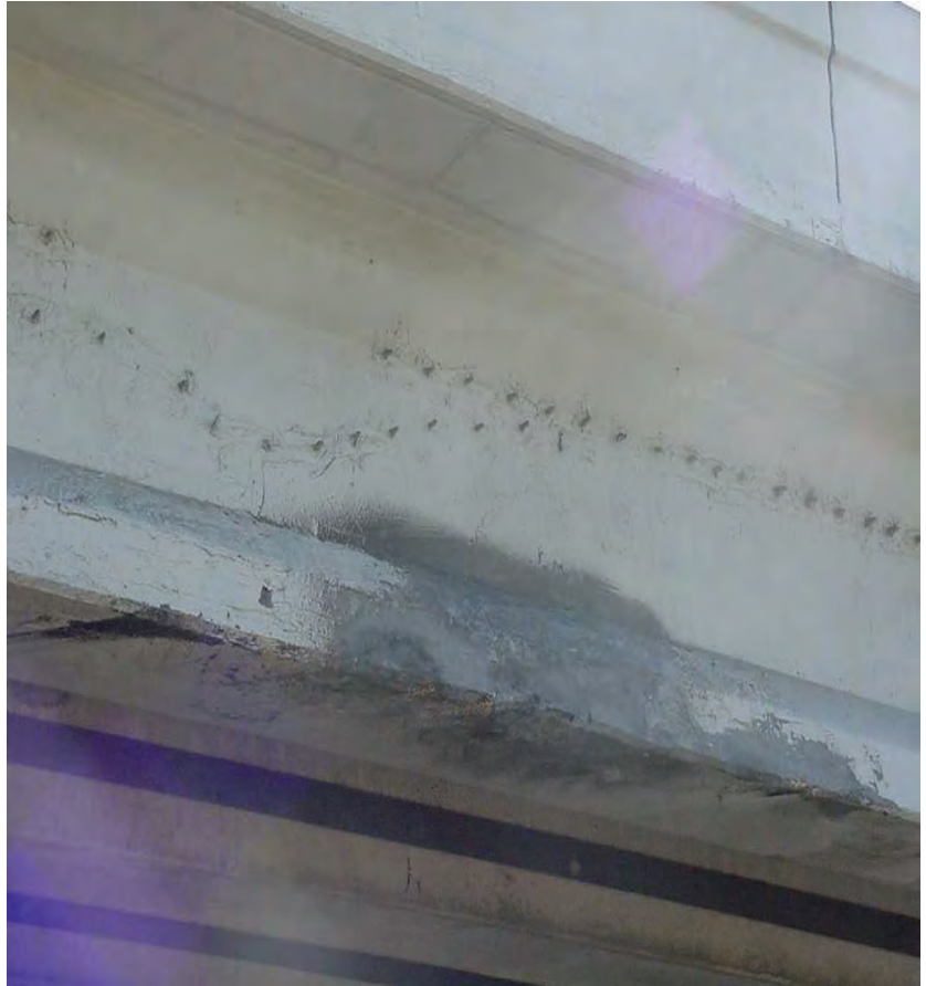
Figure 7.9.15 Collision Damage Repair on Prestressed Concrete I-beam. Note Epoxy Injection Ports
