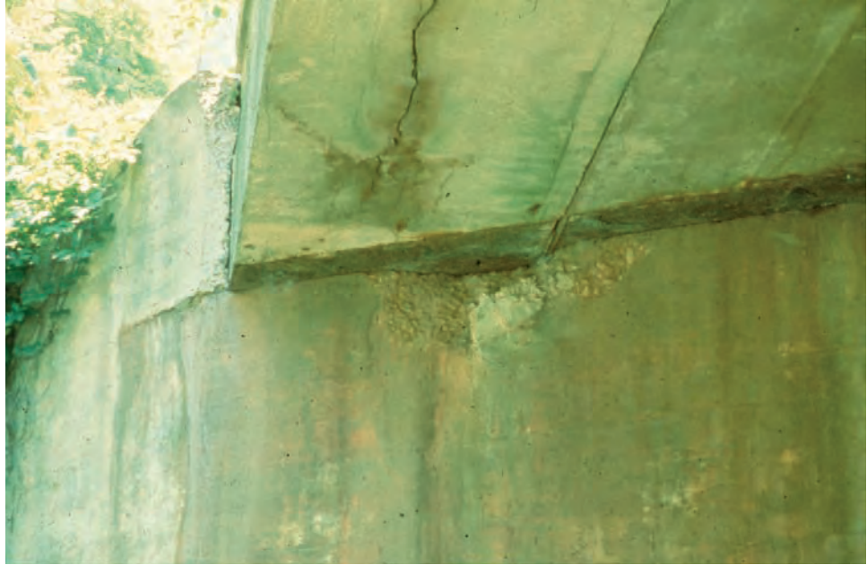
Figure 7.10.13 Longitudinal Cracks in Bottom Flange of Beam
