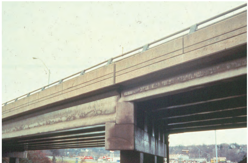
Figure 7.9.13 Leakage of Water at Joint between Spans
