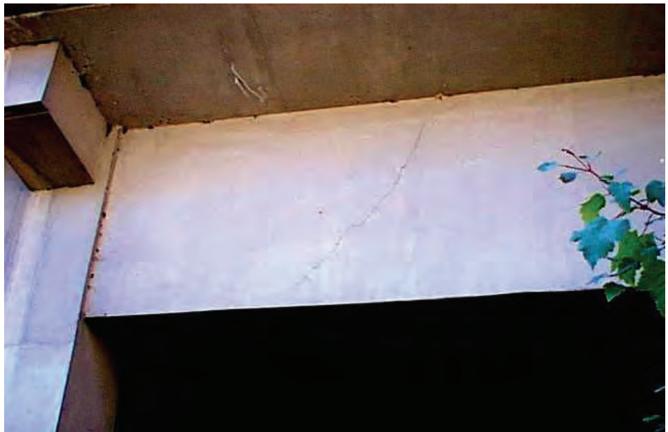
Figure 7.10.14 Diagonal Shear Crack in Web of Beam
