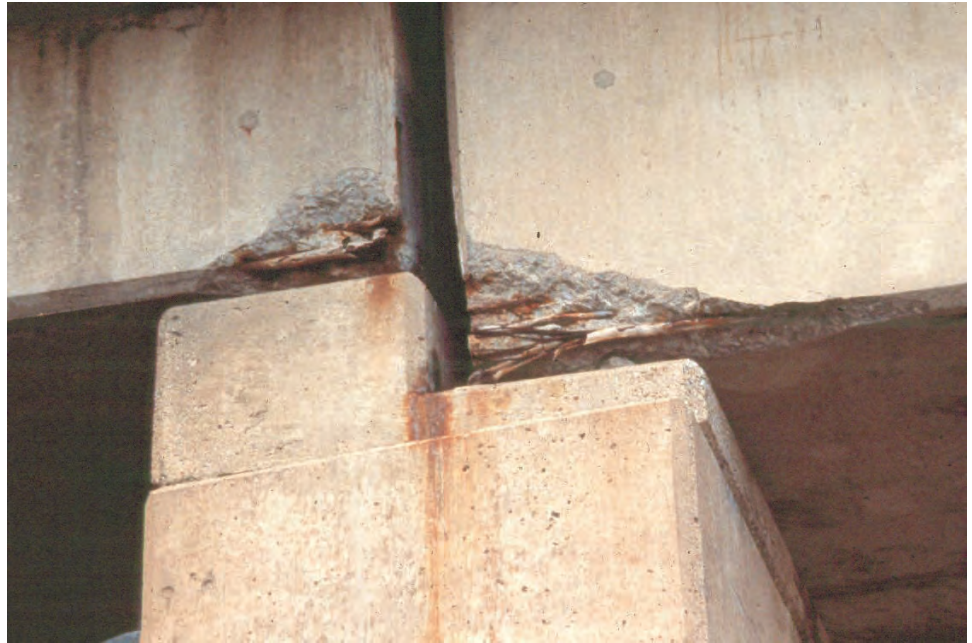
Figure 7.10.11 Spalled Beam Ends
