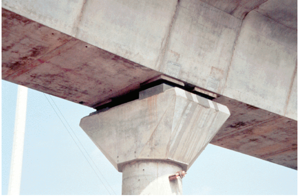
Figure 7.11.39 Segmental Box Girder Bearings at Intermediate Pier
