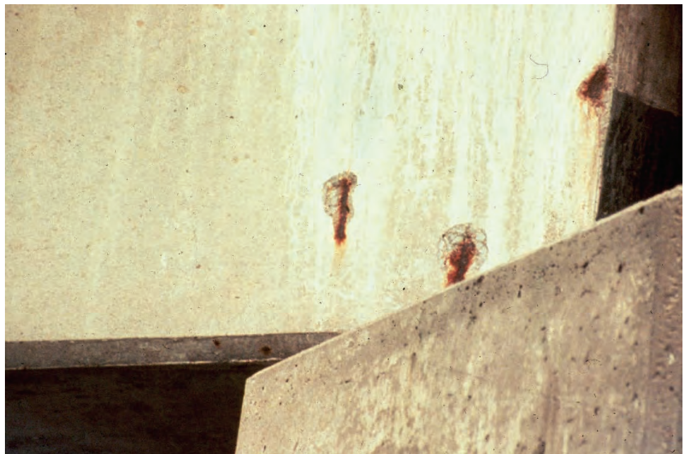
Figure 7.10.12 Exposed Bars at End of Box Beam
