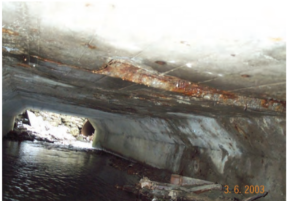
Figure 7.12.10 Spalls and Delaminations
