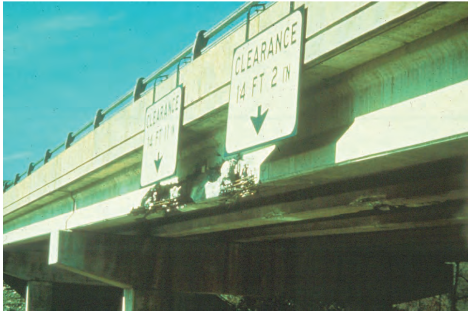
Figure 7.9.14 Collision Damage on Prestressed Concrete I-beam
