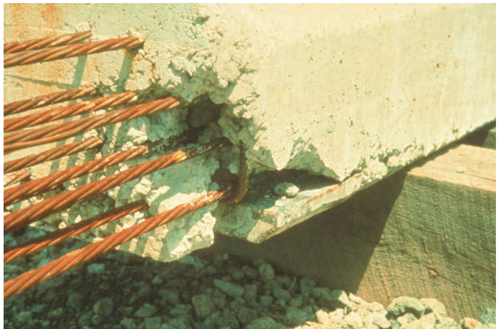
Figure 7.9.10 Spalling Due to Poor Concrete
