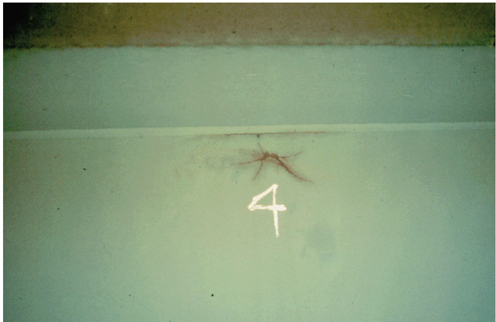
Figure 8.1.39 Through Crack in the Web
