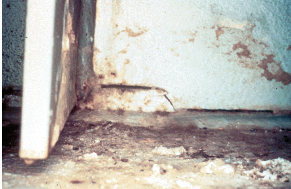
Figure 8.1.40 Through-Crack Ready to Propagate into the Flange
