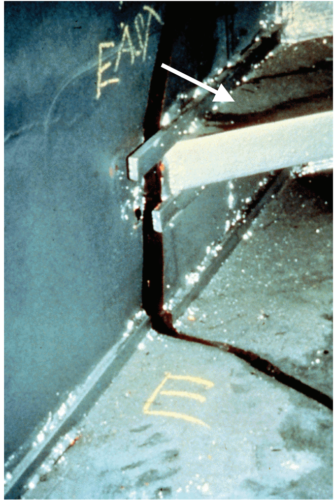
Figure 8.1.43 Poor Quality Welds Inside Cross Girder
