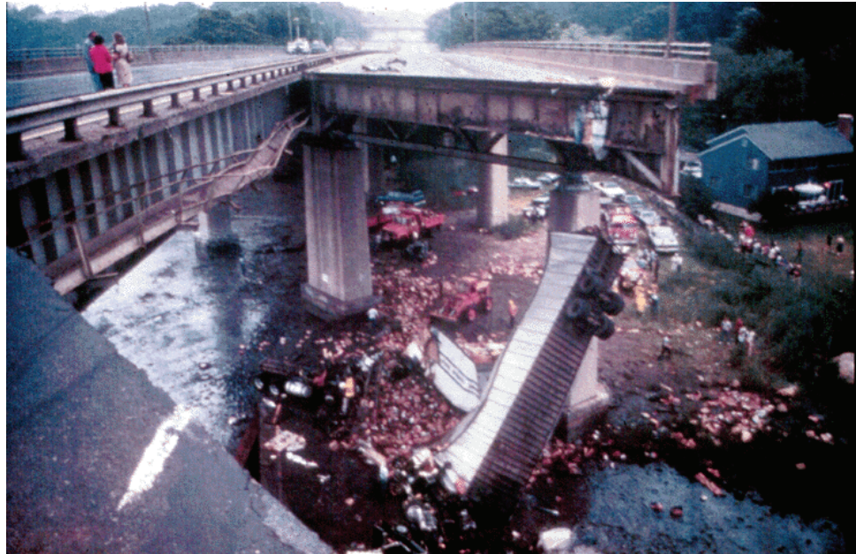
Figure 8.1.2 Mianus River Bridge Failure
