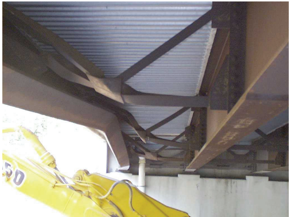
Figure 8.1.28 Severe Collision Damage on a Fascia Girder
