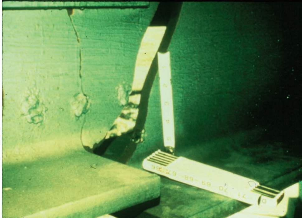
Figure 8.1.23 Crack Resulting from Plug Welded Holes
