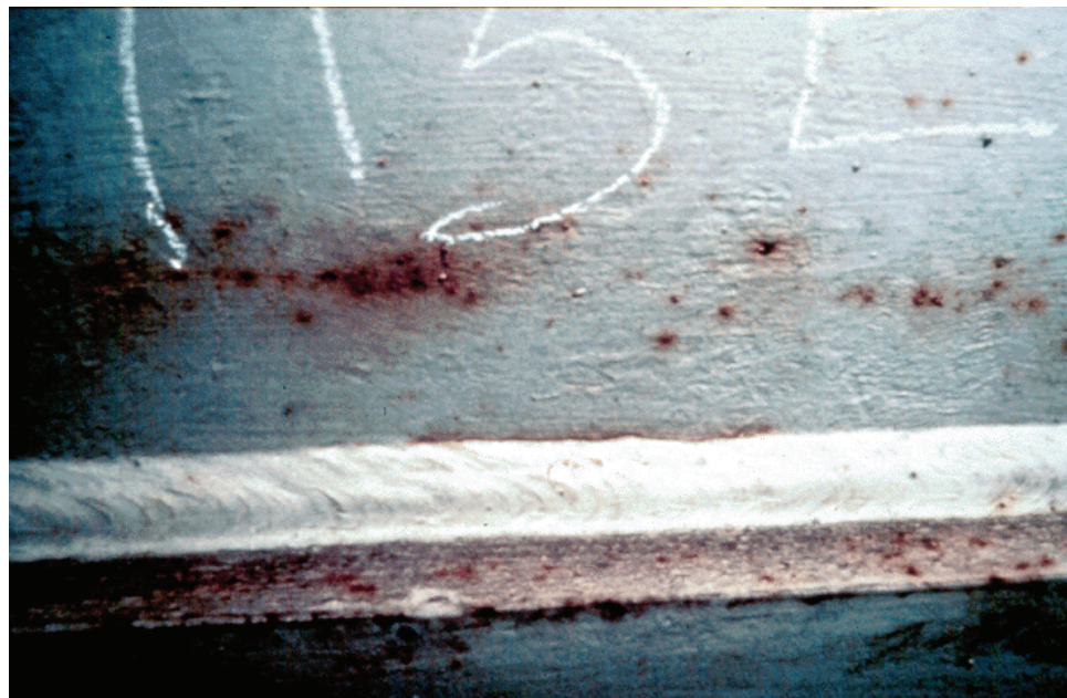
Figure 8.1.31 Part-Through Crack at a Cover Plated Flange
