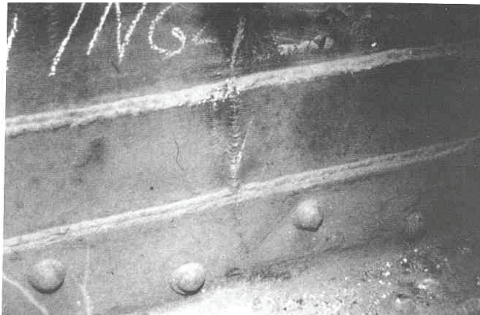
Figure 8.1.7 Patch Plate on Girder Web along Flange Angle
