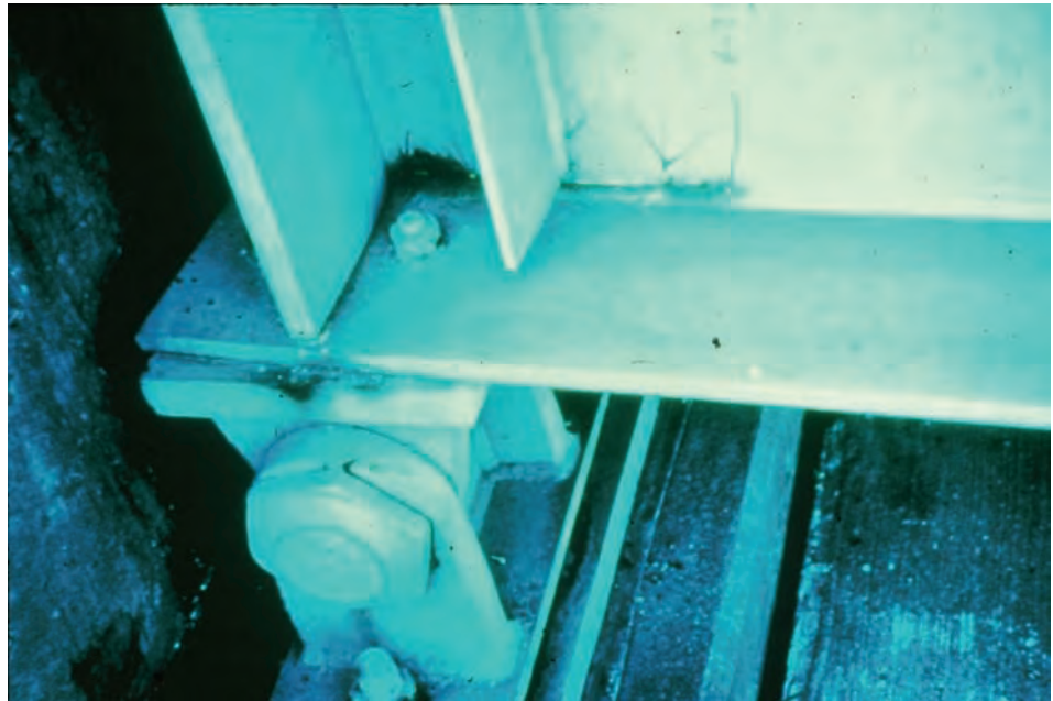
Figure 8.2.29 Web Crack due to Out-of-plane Distortion at Bottom Flange
