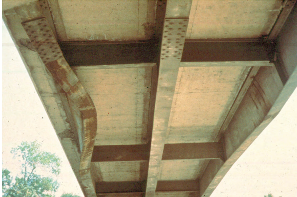
Figure 8.2.24 Collision Damage on a Fabricated Multi-girder Bridge
