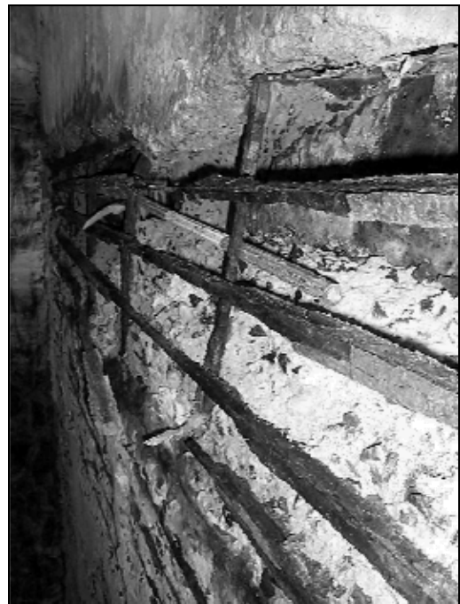
Exhibit IV. 3 Severely Deteriorated Reinforced Concrete
