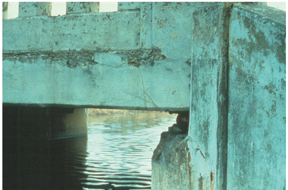
Figure 2.2.8 Shear Crack on a Slab Beam
