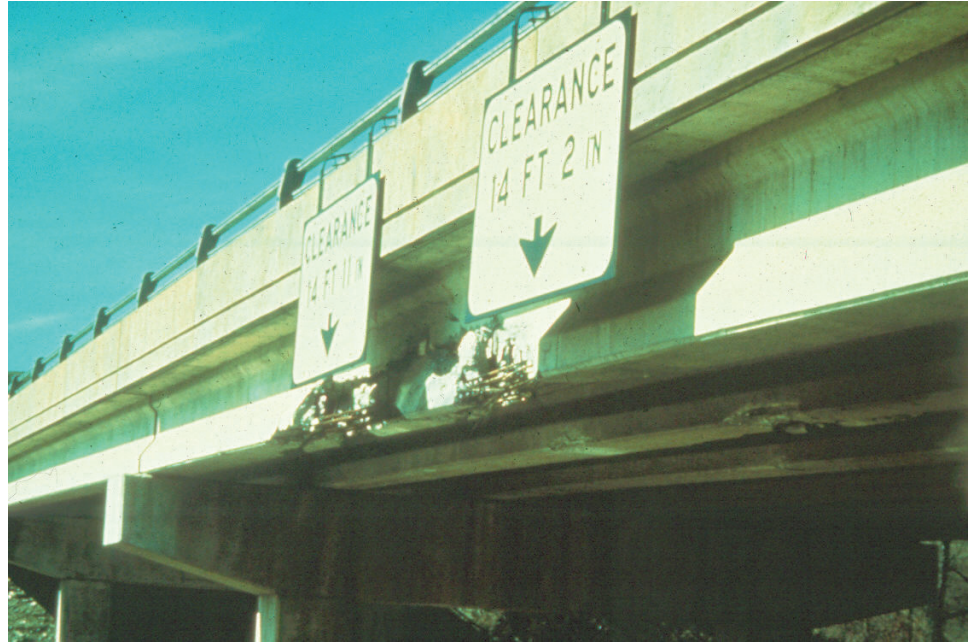
Figure 2.2.24 Collision Damage to Prestressed Concrete I-Beam
