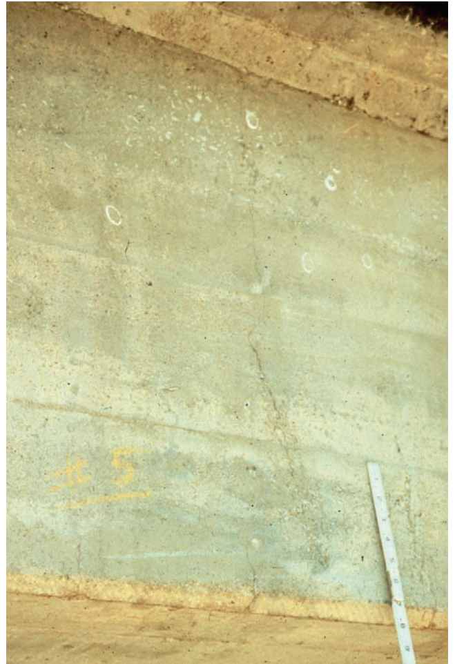
Figure 2.2.7 Flexural Crack on a Tee Beam
