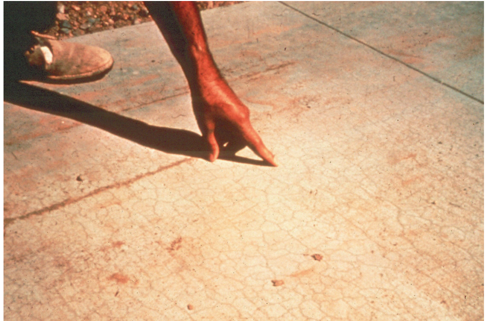
Figure 2.2.15 Pattern or Map Cracks
