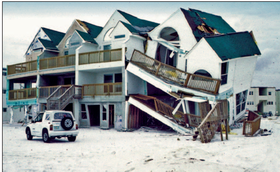
Figure 4-8. Flood and debris damage to new construction in Zone A (Hurricane Opal, 1995)
