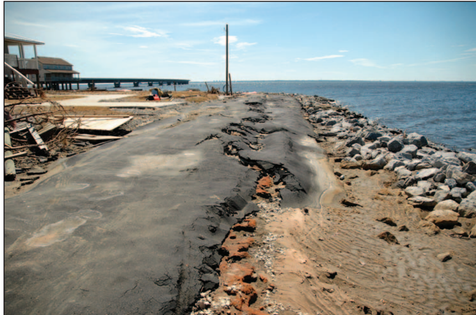
Figure 4-11. Roads placed near shorelines can wash out, causing access problems for homes such as these located at Garcon Point, FL (Hurricane Ivan, 2004)
