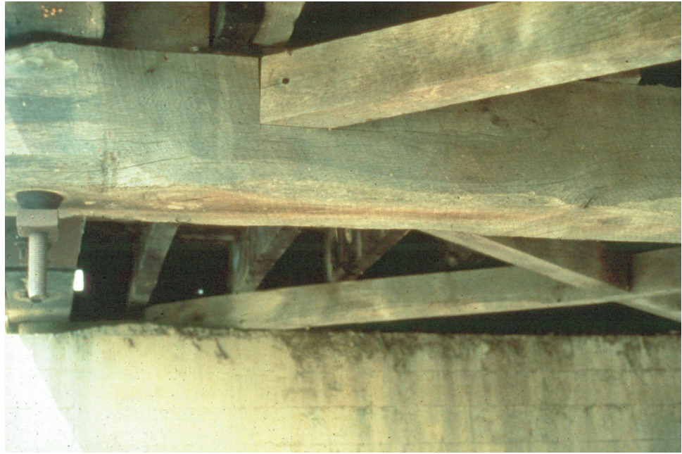
Figure 2.1.18 Loose Hanger Connection Between the Timber Truss and Floorbeam
