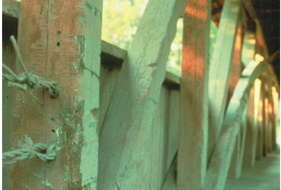
Figure 2.1.20 Impact/Collision Damage to a Timber Member
