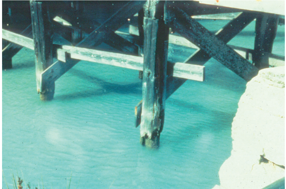
Figure 2.1.14 Marine Borer Damage to Wood Piling
