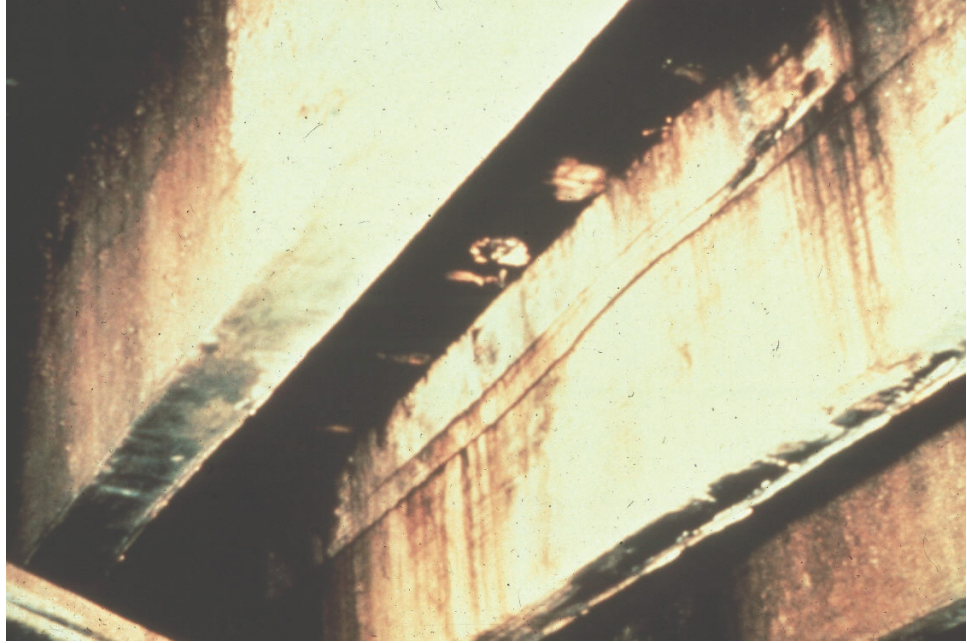
Figure 2.1.22 Horizontal Shear Failure in Timber Member
