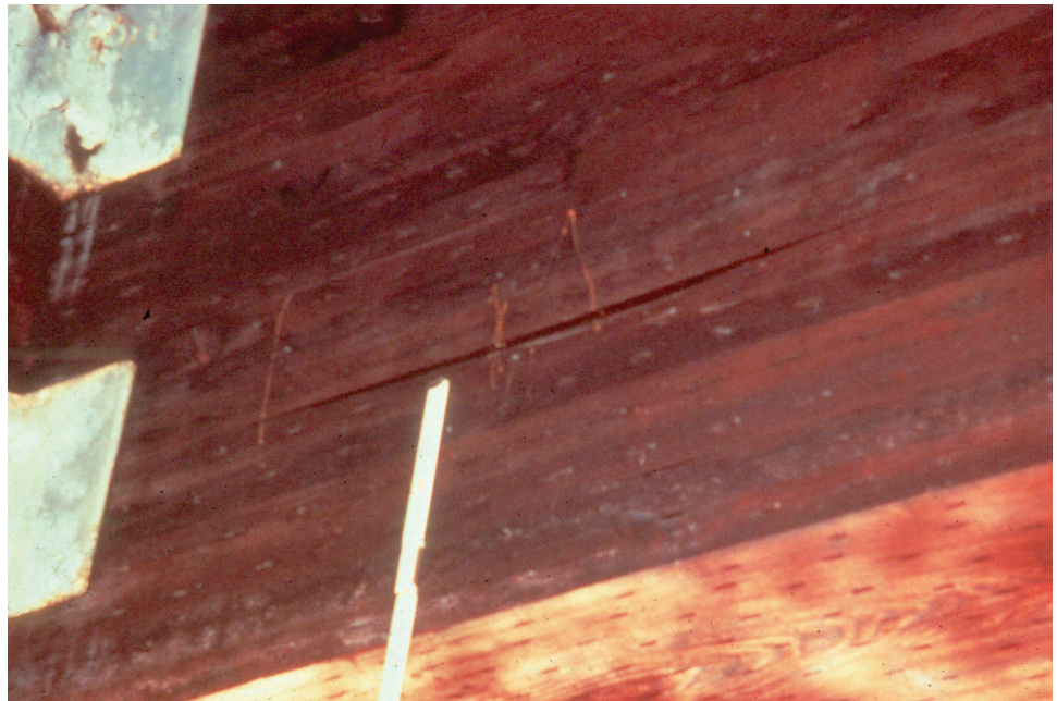
Figure 2.1.17 Delamination in a Glue Laminated Timber Member
