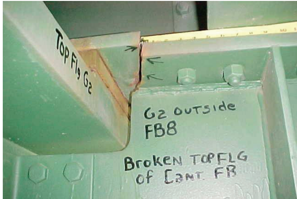
Figure 8.3.28 Cracked Cantilever Floorbeam
