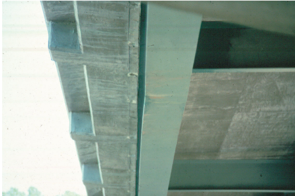
Figure 8.3.18 Collision Damage to a Two Girder Bridge
