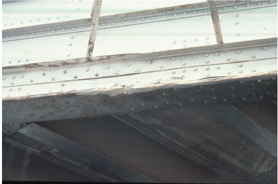
Figure 8.3.19 Collision Damage to a Through Girder Bridge
