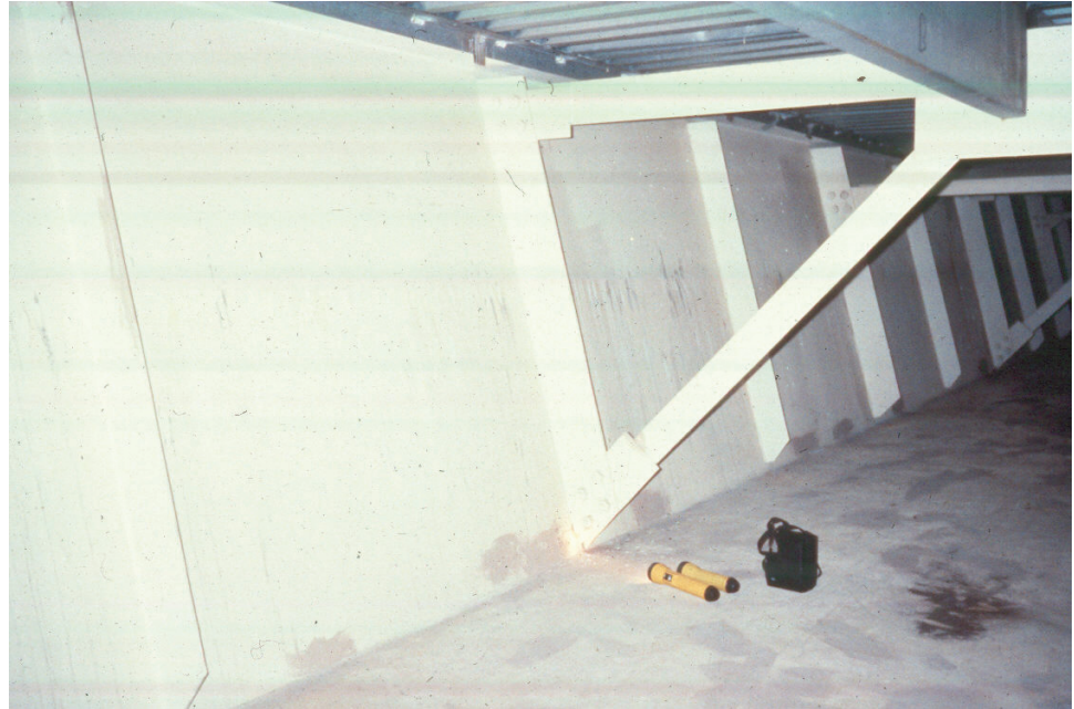
Figure 8.5.16 Box Girder Internal Diaphragm Not Attached to Flange
