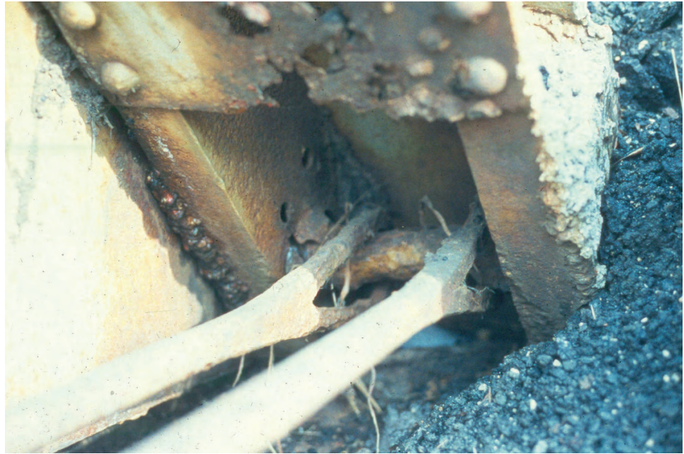
Figure 8.6.63 Worn and Corroded Pin
