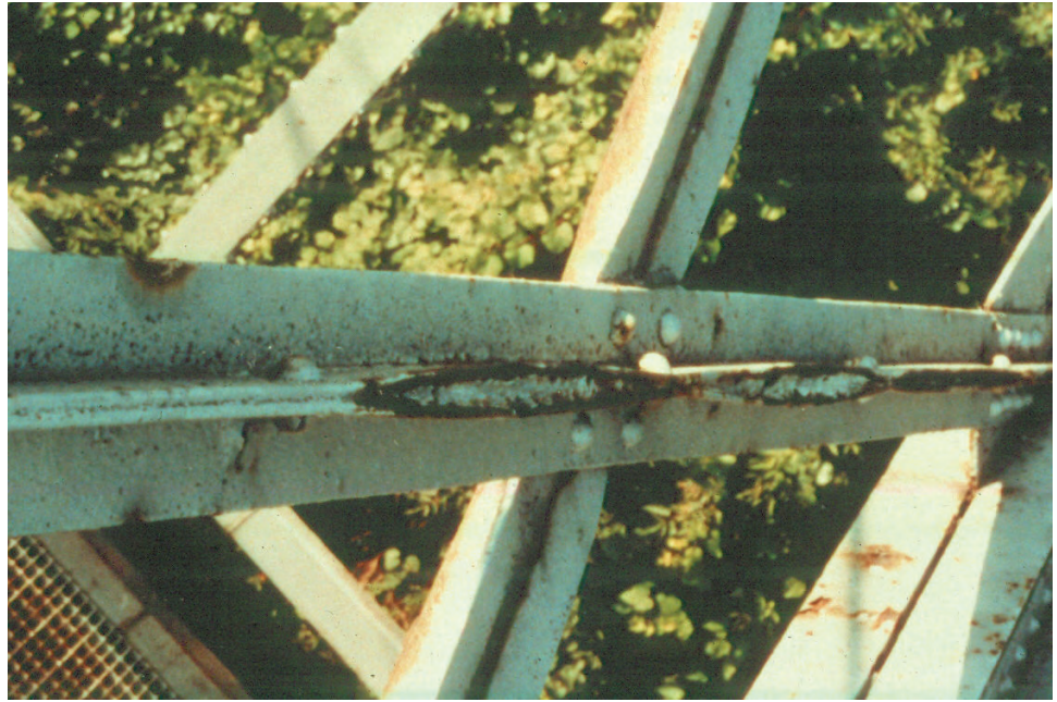
Figure 8.6.66 Sway Bracing with Rust Packing
