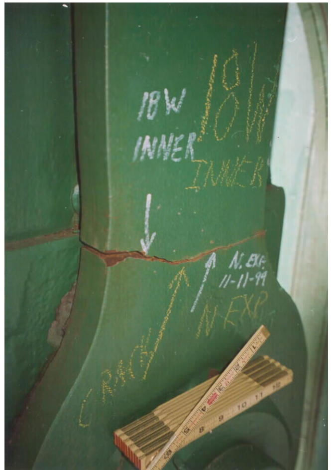
Figure 8.6.45 Cracked Forge Zone on an Eyebar
