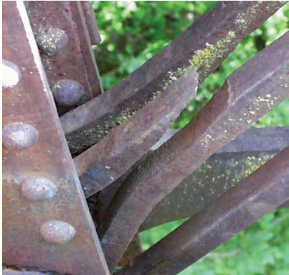
Figure 8.6.46 Cracked Forge Zone on a Loop Rod
