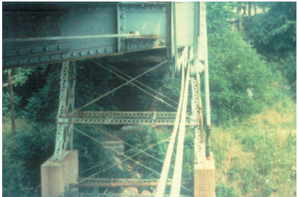
Figure 8.6.49 Bowed Bottom Chord Eyebar Member
