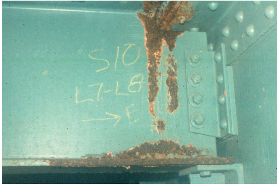
Figure 8.6.55 Corroded Stringer Connection
