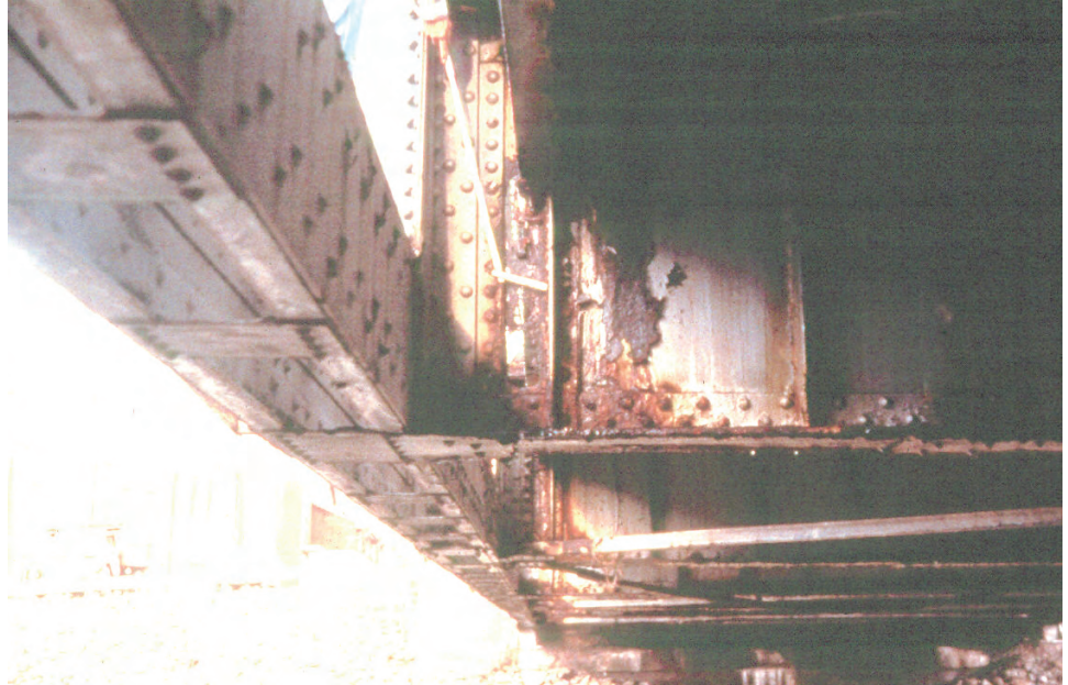
Figure 8.6.53 Corroded Floorbeam End and Connection
