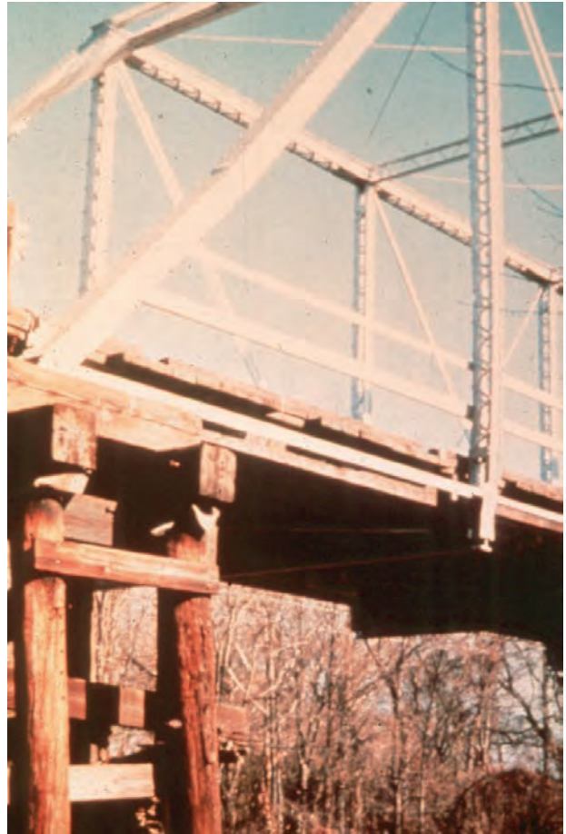
Figure 8.6.52 Buckled End Post and Temporary Supports
