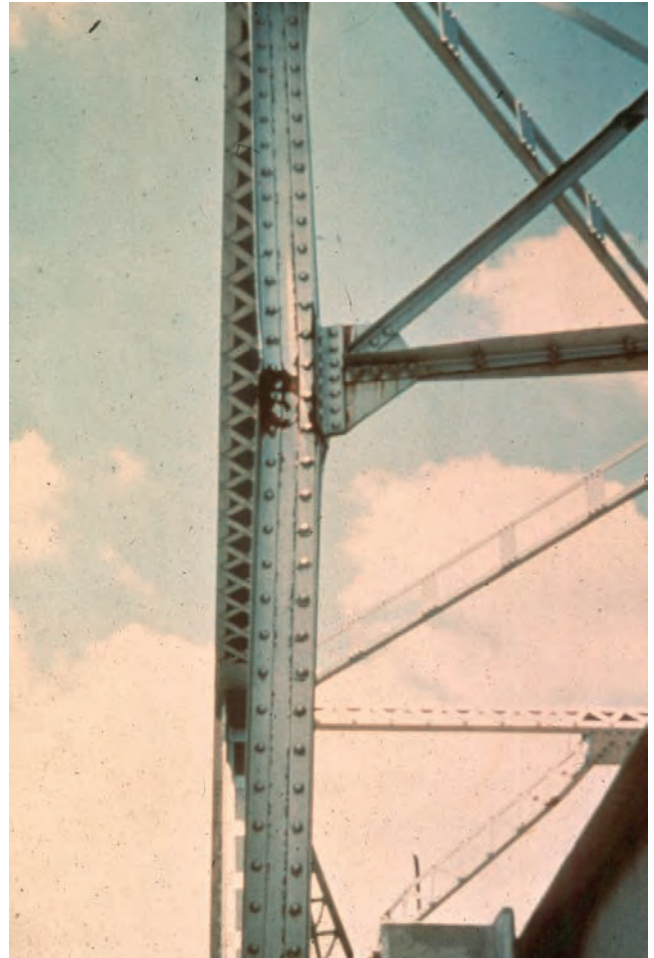
Figure 8.6.51 Collision Damage to Vertical Member
