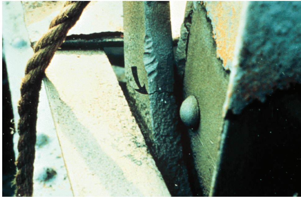
Figure 8.7.19 Close-up of the Forge Zone on an Eyebars (Arrow denotes crack)
