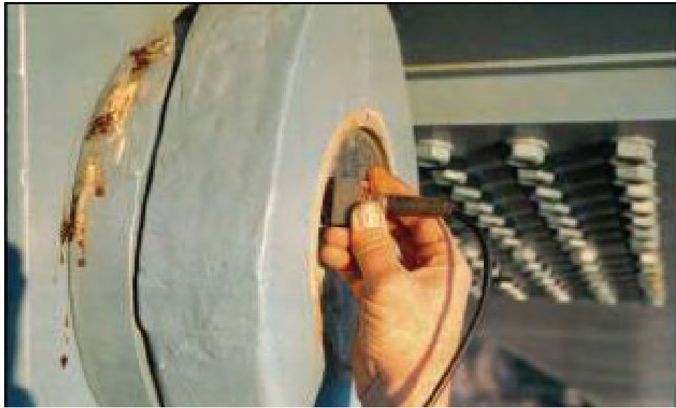
Figure 8.7.30 Ultrasonic Inspection of Eyebars Pin
