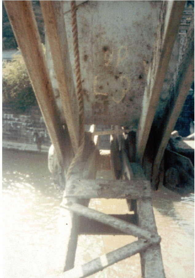
Figure 8.7.15 Loosely Packed Eyebar Connection
