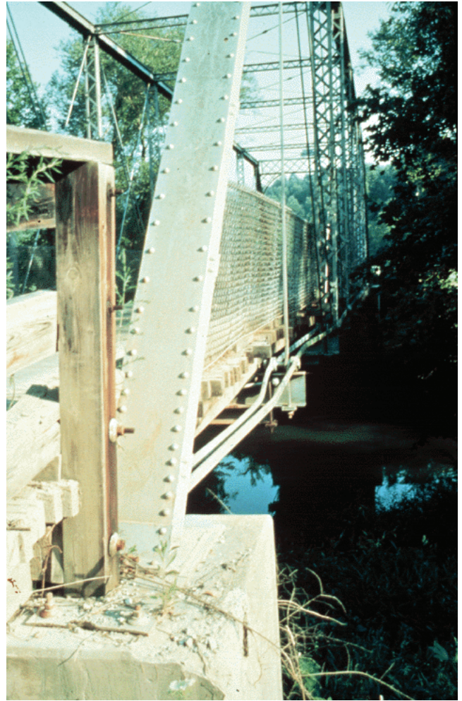
Figure 8.7.21 Buckled Eyebar due to Abutment Movement
