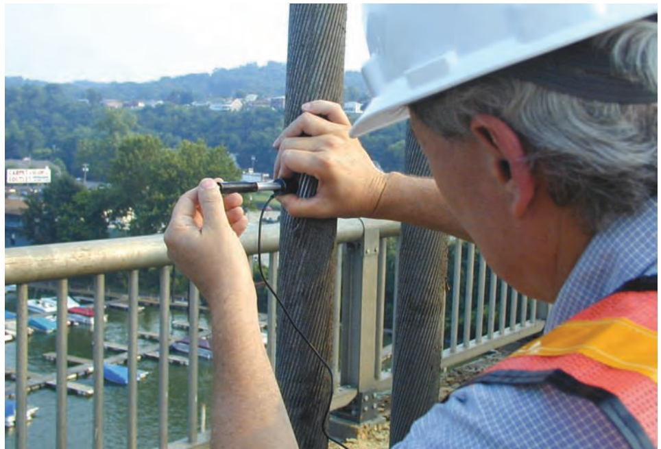
Figure 8.8.20 Performing Baseline Hardness Test on Fire Damaged Arch Cables
