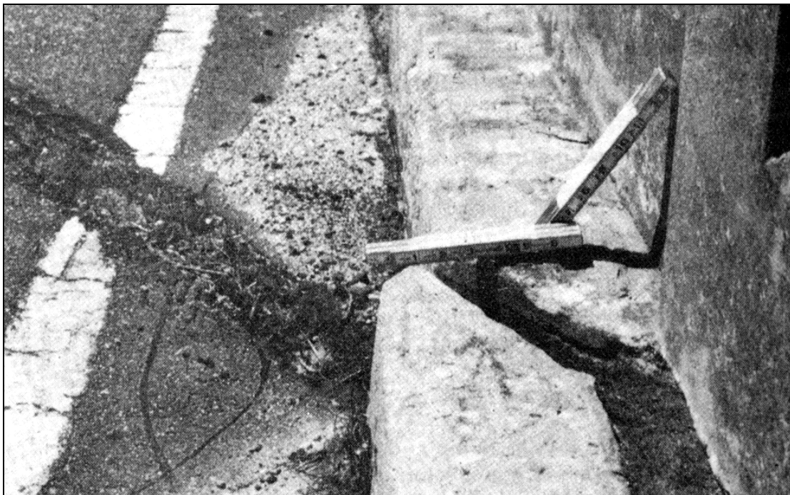
Exhibit X.26 Joint Filled with Debris
