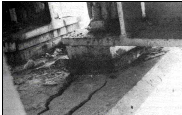
Exhibit X. 25 Crack in Seat
