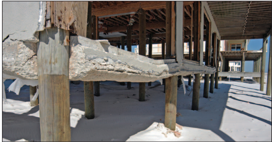
Figure 3-25. The sand underneath this Pensacola Beach, FL, building was eroded due to wave runup and storm surge (Hurricane Ivan, 2004)
