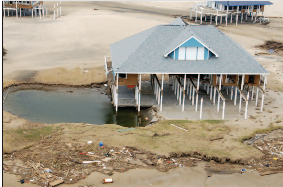
Figure 3-49. Residential foundation that suffered severe scour on Bolivar Peninsula, TX (Hurricane Ike, 2008)
