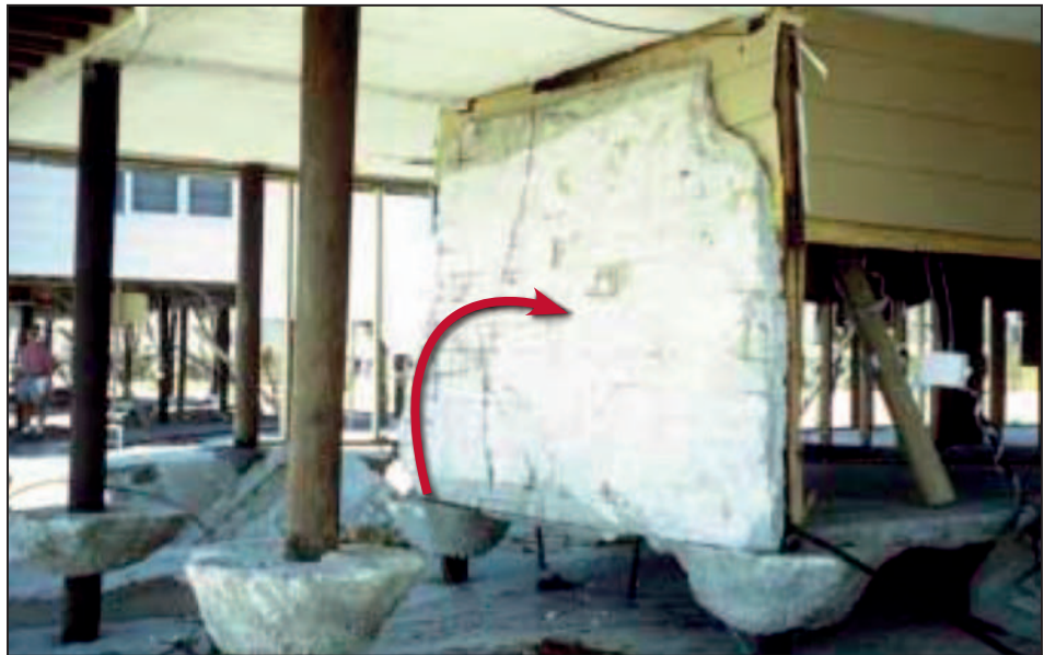
Figure 3-26. Concrete slab-on-grade flipped up by wave action came to rest against two foundation members, generating large unanticipated loads on the building foundation (Topsail Island, NC, Hurricane Fran, 1996)
