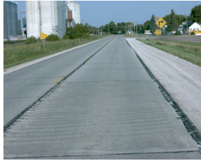
Rumble warning panel
