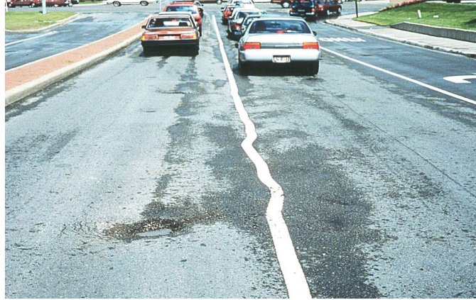
d) Drainage problems
