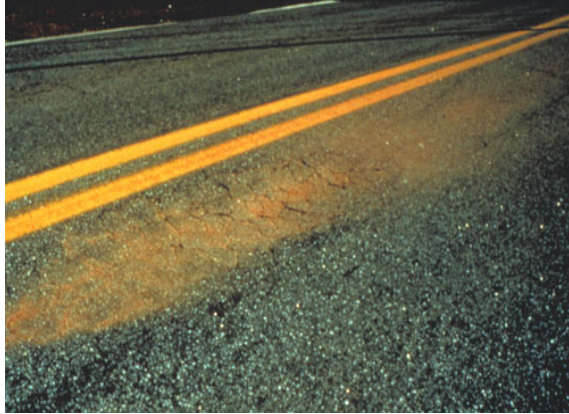
c) Subgrade pumping
