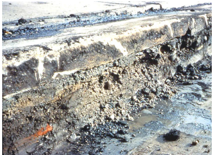
b) Aggregate contamination or degeneration
