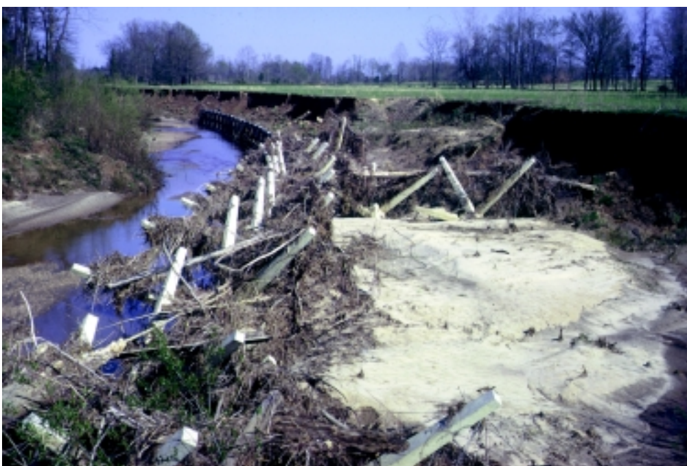
Figure 16-31 Concrete jack system several years after installation
