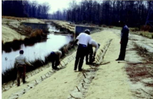
Figure 16-9b Installing live stakes in live fascine system (Robbin B. Sotir & Associates photo)
