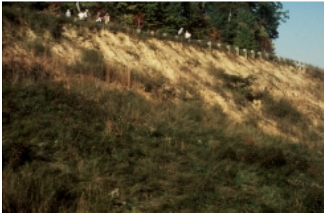
Figure 18-1a Eroding fill slope
