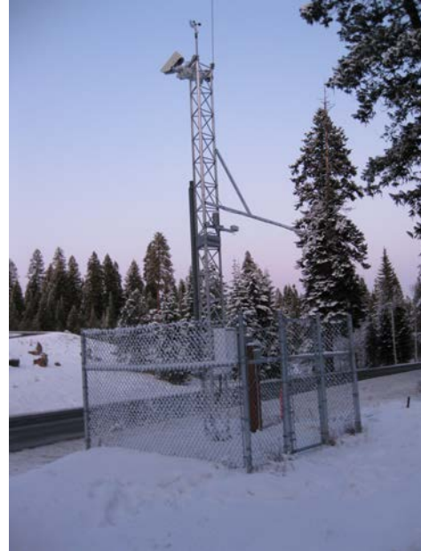
Figure ID-1. RWIS installation at Goose Creek Summit on State Highway 55 in central Idaho.
