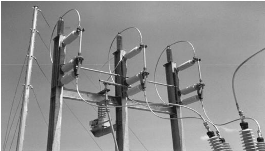
Figure 5.-25: Vertically Mounted Vertical-Break Switch. Courtesy of Tuley & Associates, Inc.
