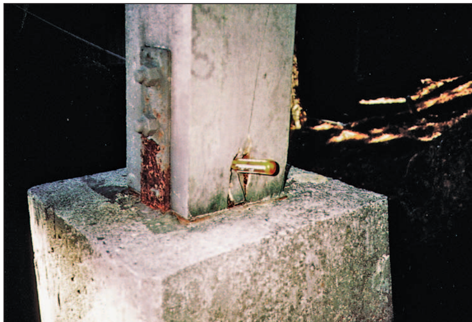
Figure 13-9. Wood decay at the base of a post supported by concrete
