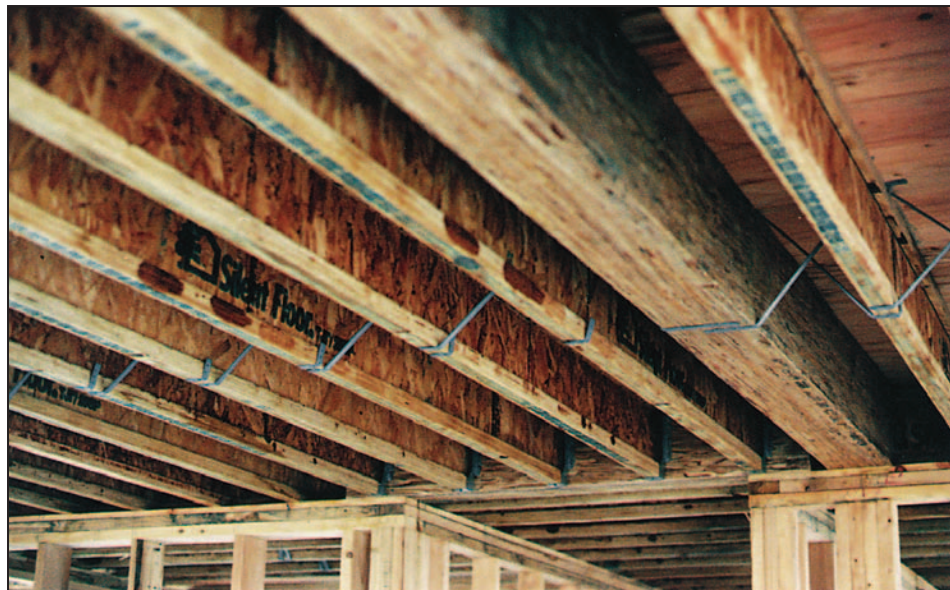
Figure 13-20. Engineered joists used as floor joists with proper metal brace to keep the bottoms of the joists from twisting; engineered wood beam
