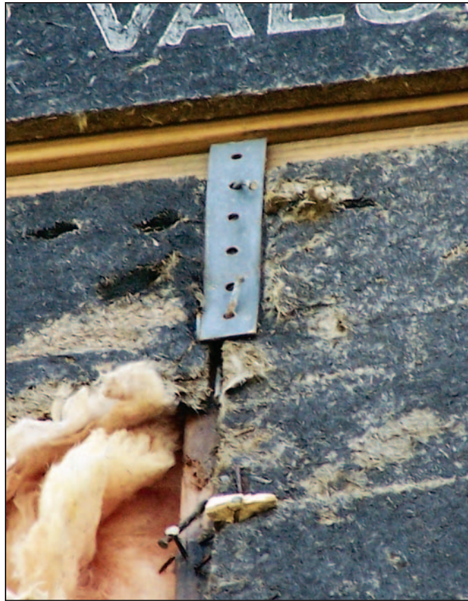
Figure 13-15. Connector failure caused by insufficient nailing
