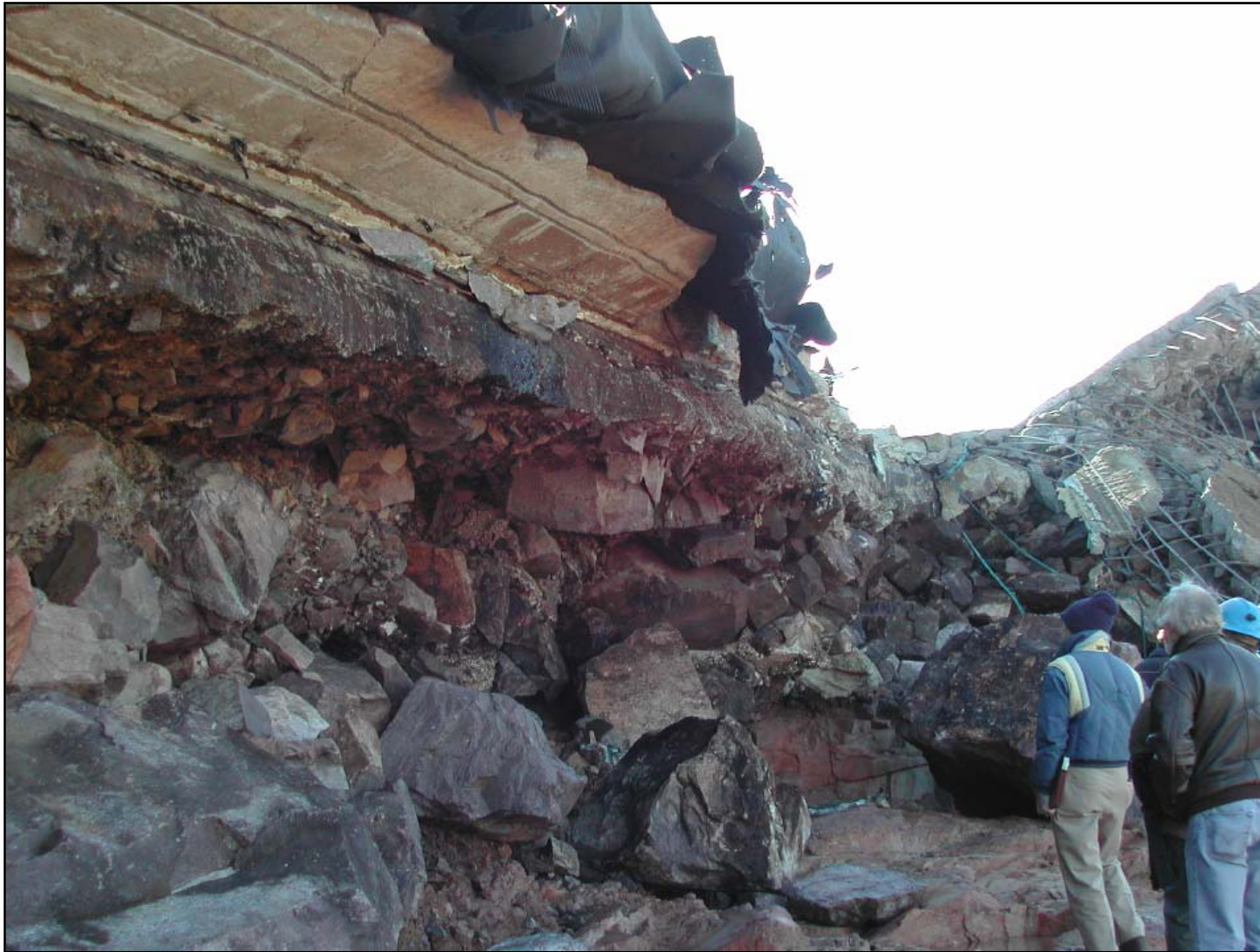
Rockfill between top of rock and base of plinth, note reddish grout in rockfill beneath the plinth
