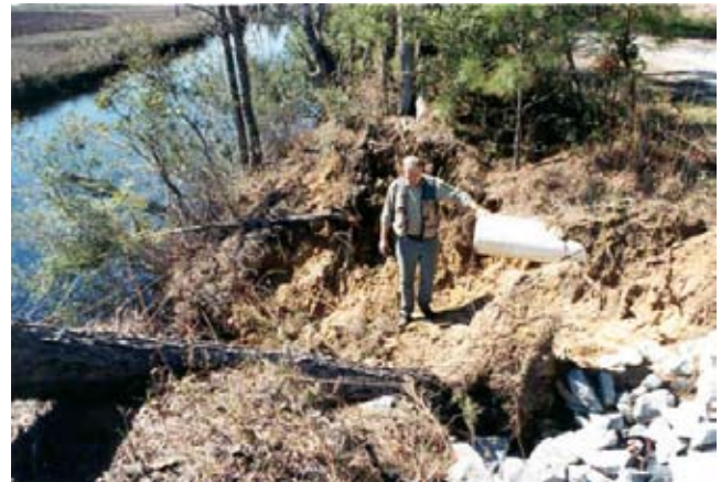
Figure TS14P-10 Slope failure due to excessive runoff from a road
