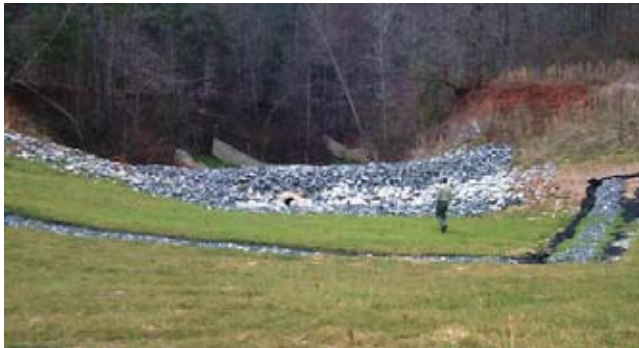
Figure TS14P-28 Reshaped gully with terrace failure, Abbeville County, SC
