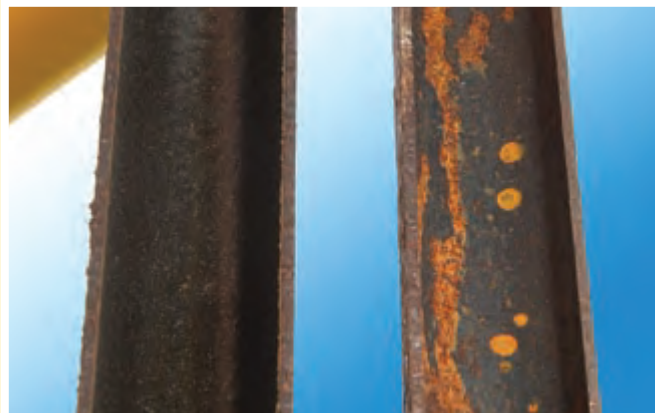
PPS coating on the left and a failed coating on the right.
