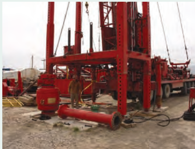
Wellhead with spool and blowout preventer in foreground at Raft River.
