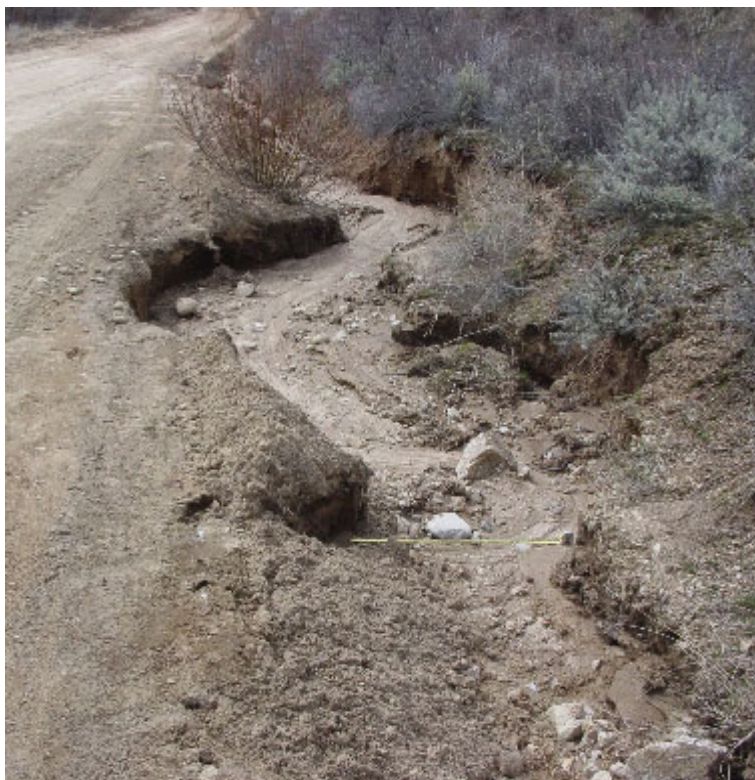
Figure 7-17 — Example of an inadequate ditch eroding shoulder material.
