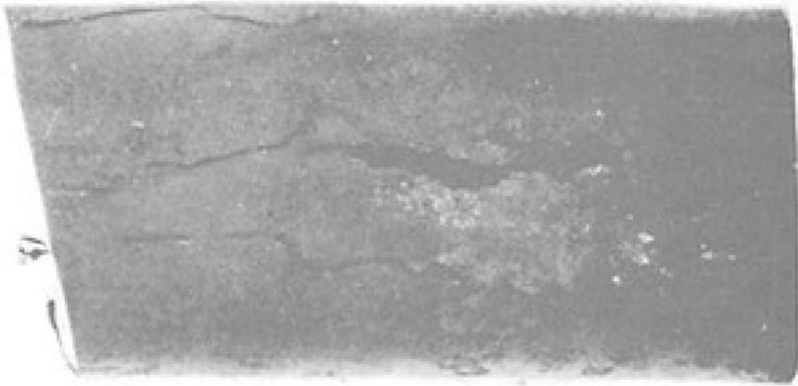
Figure 8-18 — Thermal crack in a superheater tube.
