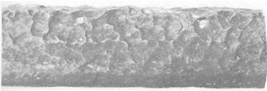
Figure 8-12 — General fireside thinning of a stainless steel superheater tube (results of fuel ash damage).
