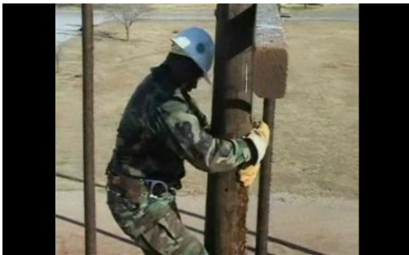
Figure 4-13 – Individual descending utility pole.
