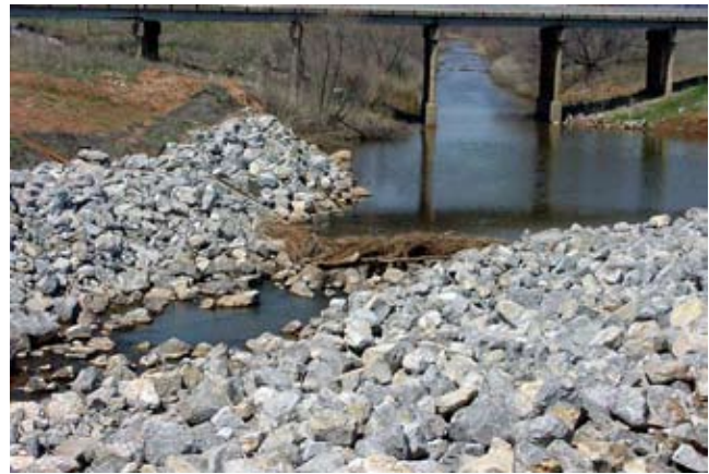
Figure TS14C-3 Riprap used to prevent erosion from flow from a side inlet to a channel
