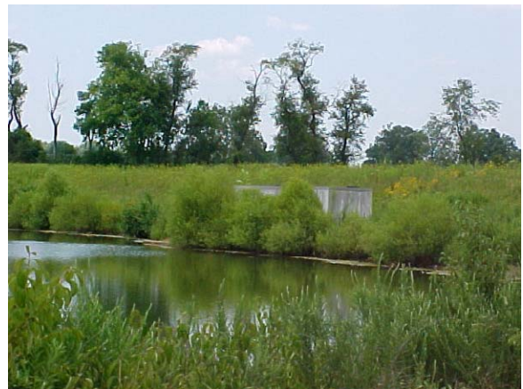
Figure 1.9: Excessive vegetative growth obscures riser
