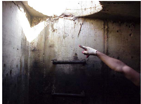
Figure M6.2: Missing manhole step.
