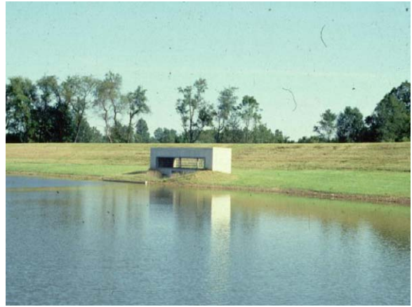
Figure M1.1: Riser located near pool edge for easier access.
