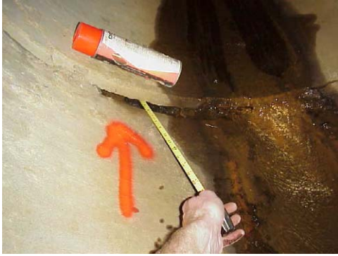
Figure 2.3: Marking pipe joint separation
