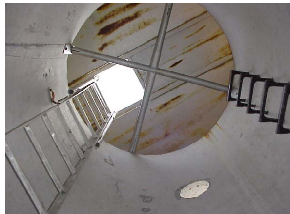
Figure 1.13: Ladder and steps in riser.
