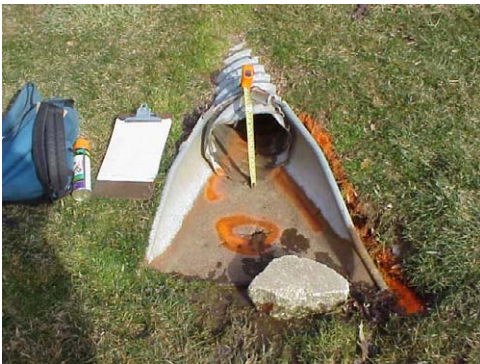
Figure 2.1: Marking outfall deficiencies.
