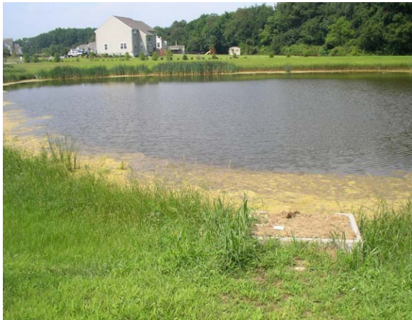
Figure 1.2: Flattop riser covered with debris.
