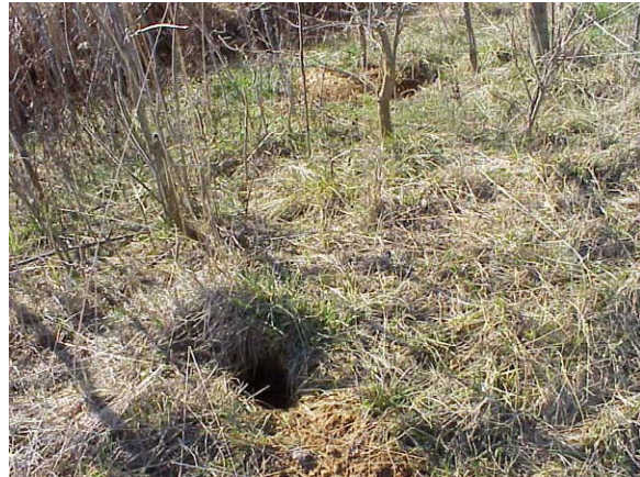
Figure M8.1: Animal burrow in pond embankment.
