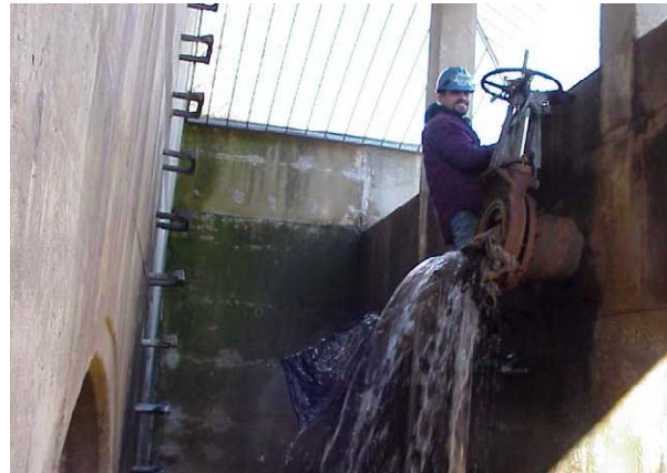
Figure M2.1: Clogged valve.
