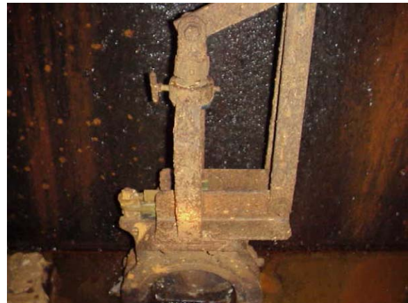
Figure 1.16: Corroded plumbing and valve.
