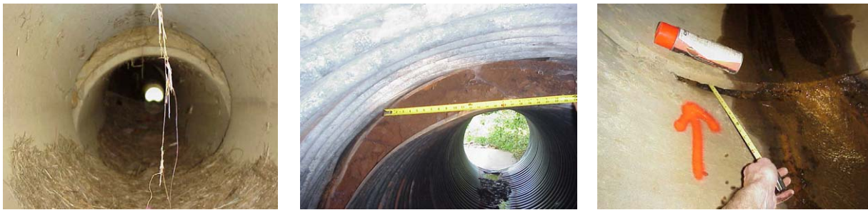
Figure M3.3: Misalignment in RCP (left and right) and CSP (center) applications.
