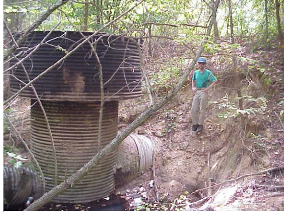
Figure 1.5: Severe erosion around riser and barrel
