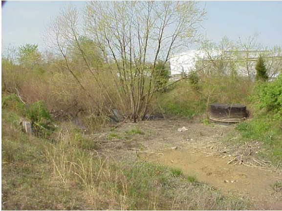
Figure 1.10: Sediment accumulation in a dry pond
