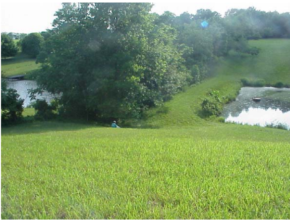
Figure 1.8: Woody vegetation on embankment
