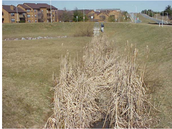
Figure M4.6: Vegetation establishment where the inflow channel slope is inadequate to drain properly.
