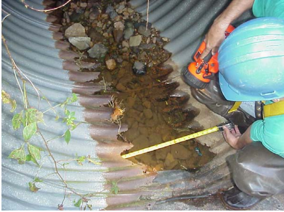
Figure 1.4: Pipe invert abrasion
