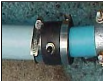
Test boot located in a sump
