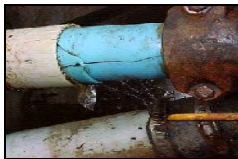
Flexible piping is cracked
