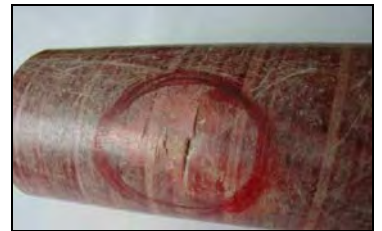
Fiberglass piping is cracked
