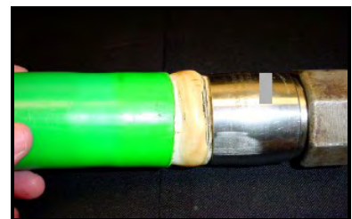
Flexible piping is bulging
