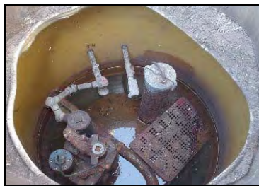
Contained sump with liquid and debris
