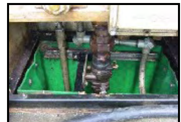
Contained dispenser sump
