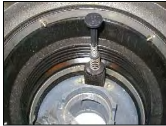
Spill bucket drain valve
