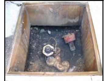
Uncontained turbine sump
