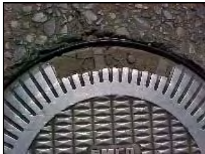
Cracked spill bucket lid
