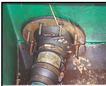
Sump penetration seals in poor condition
