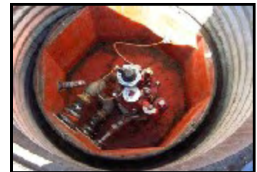
Contained turbine sump
