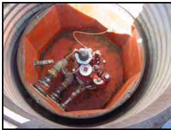
Dry, debris-free contained turbine sump
