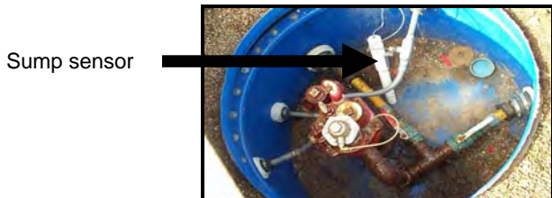
Sump sensor in contained turbine sump
