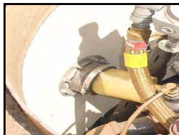
Sump penetration seals in good condition
