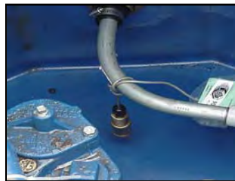
Liquid sump sensor
