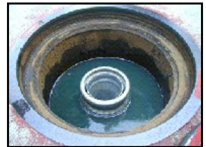
Spill bucket that contains liquid
