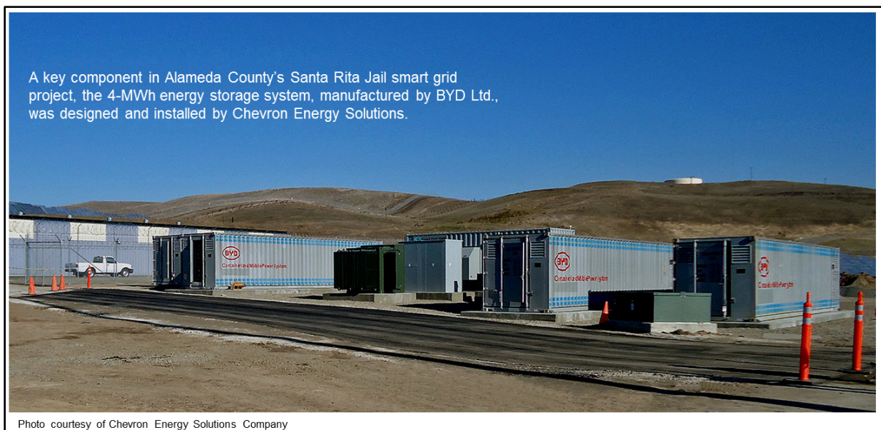
Figure 98. A 2-MW/4-MWh Li-ion Energy Storage System
