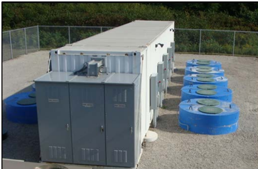
Figure 90. 1-MW Smart Energy Matrix Plant
